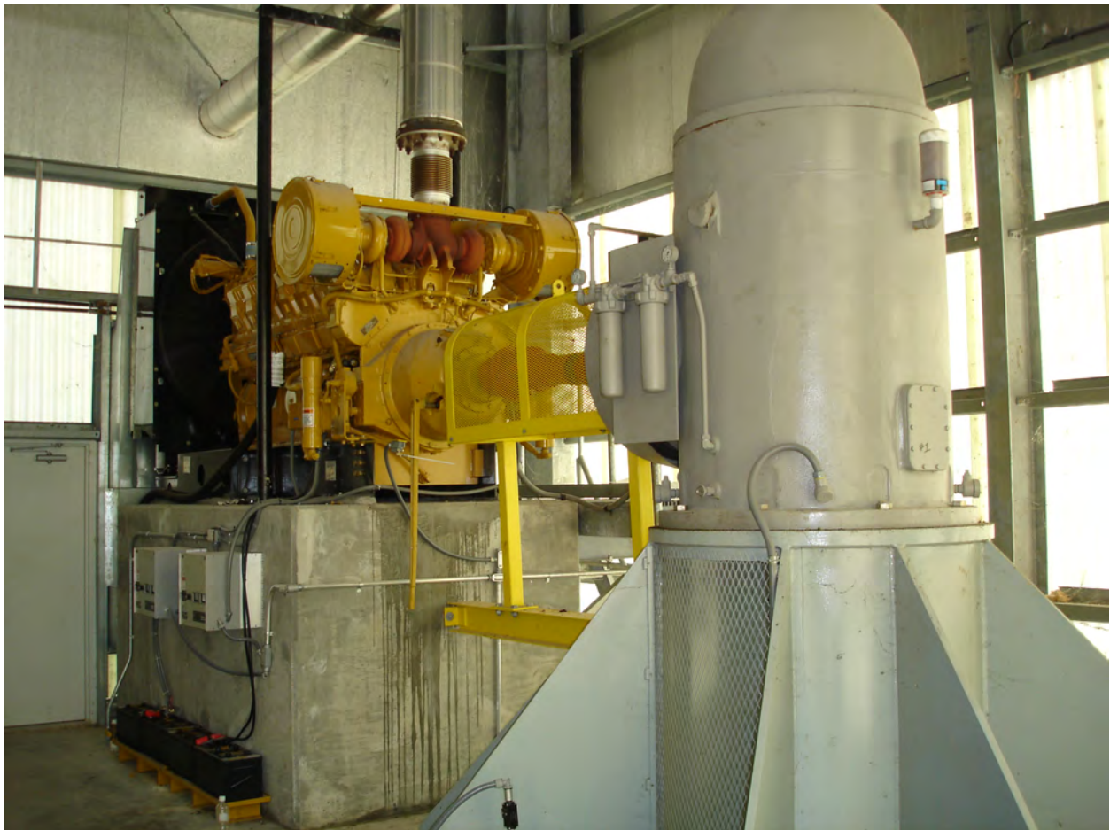
Figure 20. Vertical diesel driven pump with right-angle drive speed reducer.
