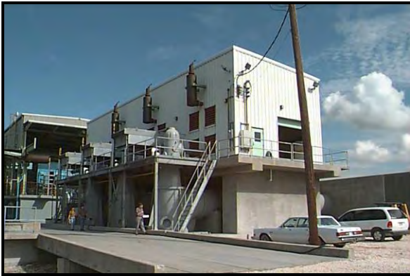
After Hurricane Katrina: View from the inlet canal
