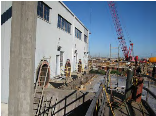
After Hurricane Katrina: View from the discharge
