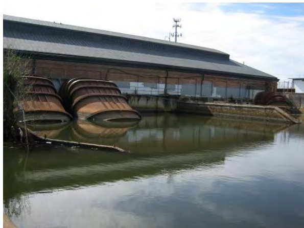
After Hurricane Katrina: View from the discharge
