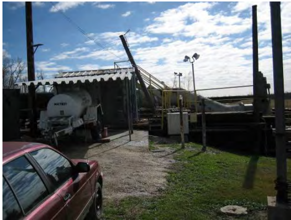
After Hurricane Katrina: View from the side
