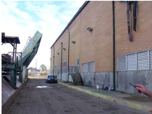
After Hurricane Katrina: View from the side of the intake canal
