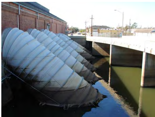
After Hurricane Katrina: View from the discharge
