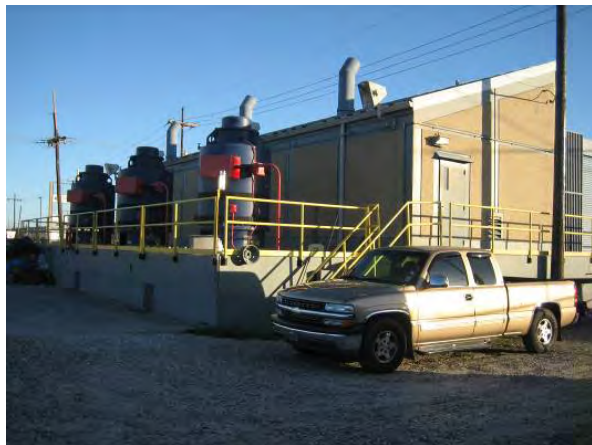
After Hurricane Katrina: View from the discharge
