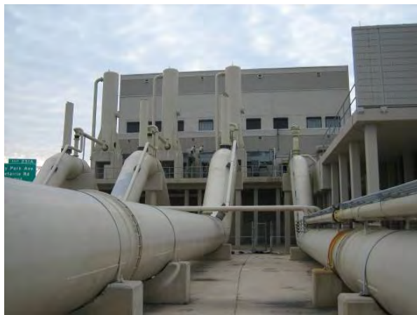
After Hurricane Katrina: View from the discharge
