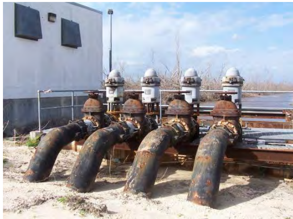
After Hurricane Katrina: View from the discharge
