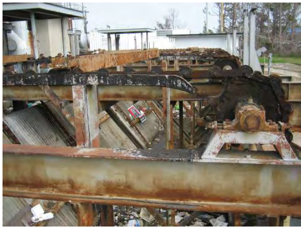
After Hurricane Katrina: View from the discharge
