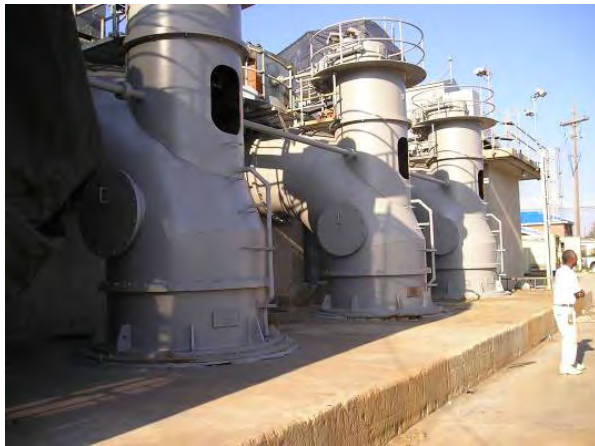
After Hurricane Katrina: View of the pumps
