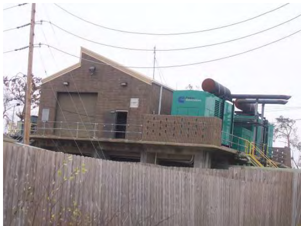
After Hurricane Katrina: View from the side
