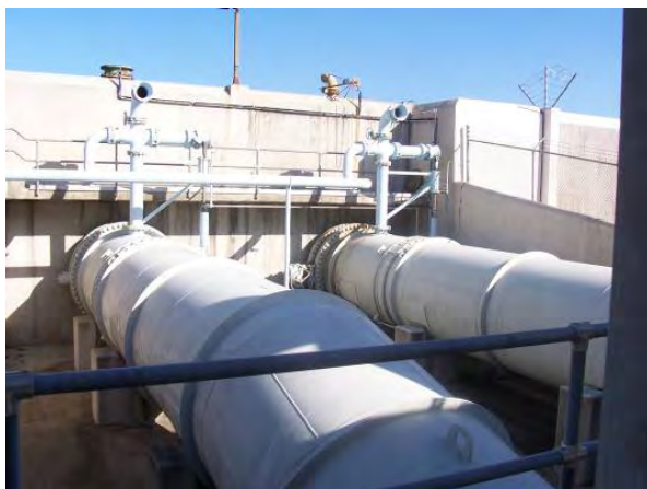
After Hurricane Katrina: View from the discharge
