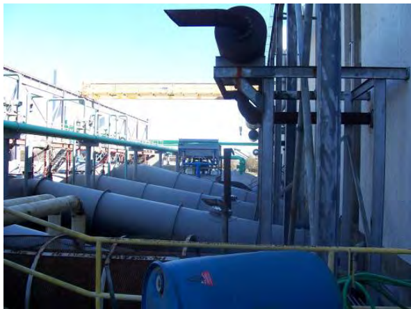
After Hurricane Katrina: View from the discharge
