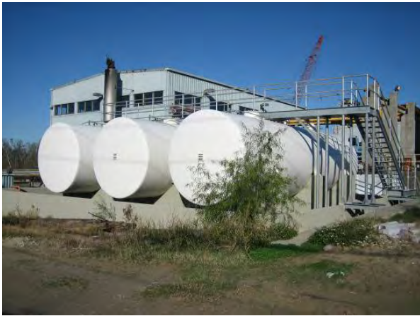
After Hurricane Katrina: View from the side
