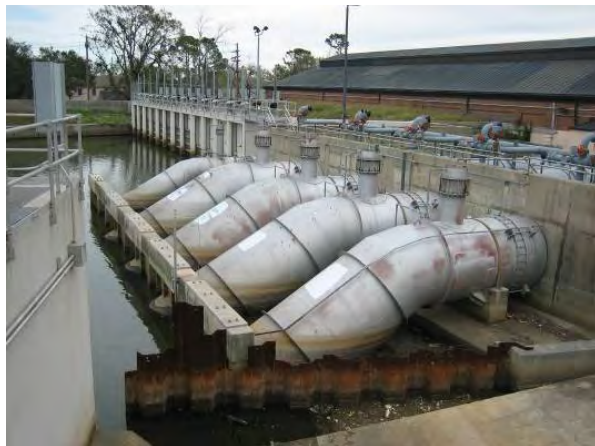
After Hurricane Katrina: View from the discharge
