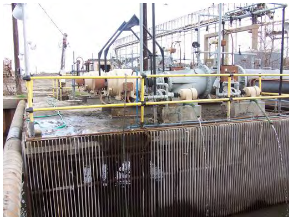
After Hurricane Katrina: View from the discharge
