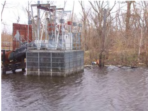
After Hurricane Katrina: View of the station
