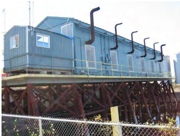
After Hurricane Katrina: View from the discharge
