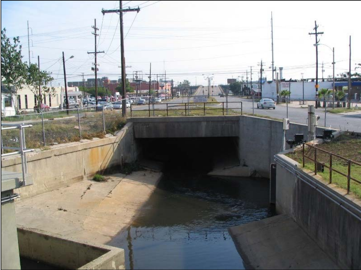
Photo 3. Broad Street Canal entering Pump Station No. 1.
