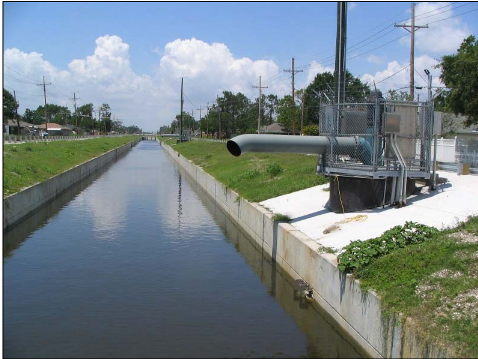
Photo 25. N. Cumberland interior pump at Interior Canal No. 4, W. Napoleon Avenue.
