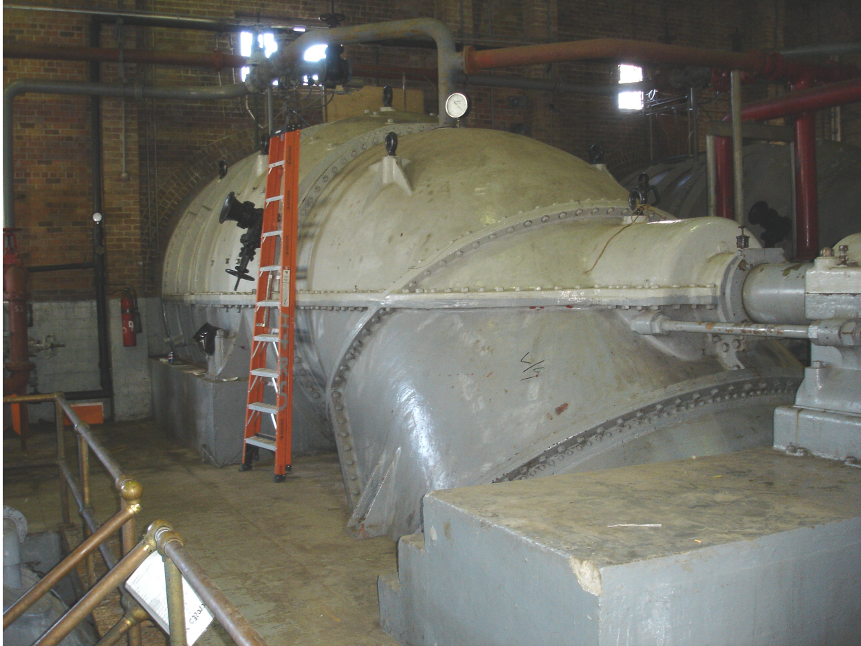
Figure 7. Large horizontal shaft pump.
