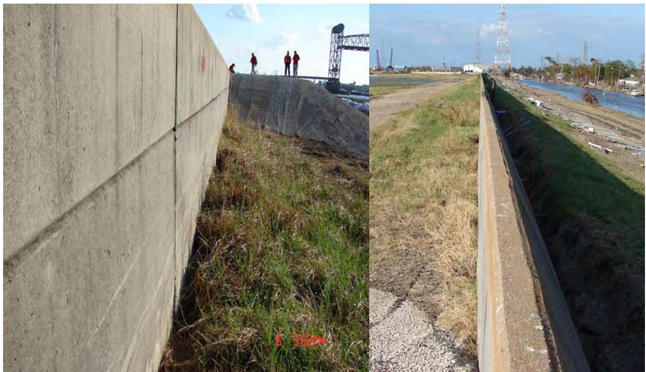
Figure 48. IHNC East Bank – South Breach – Wall Movement
