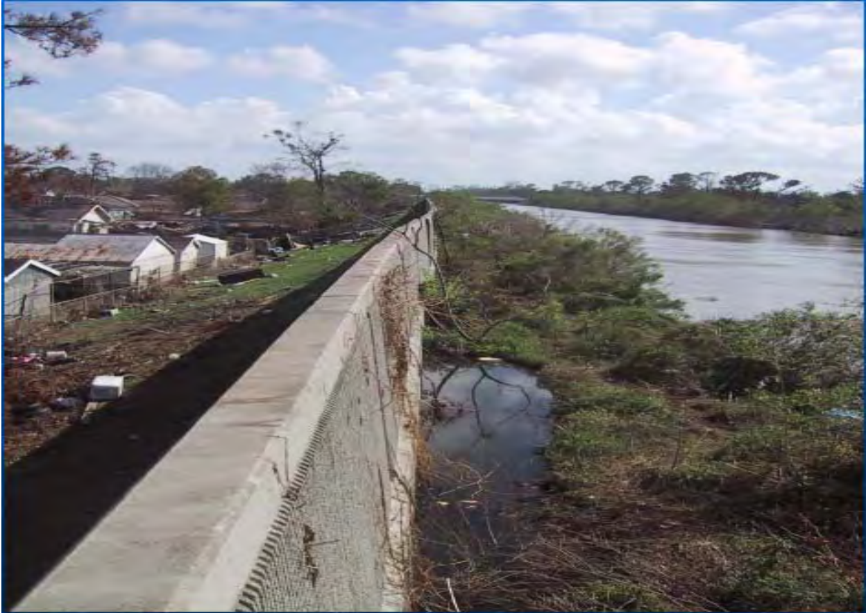
Figure 31. Tilted I-Wall Opposite the North Breach on the London Avenue Canal
