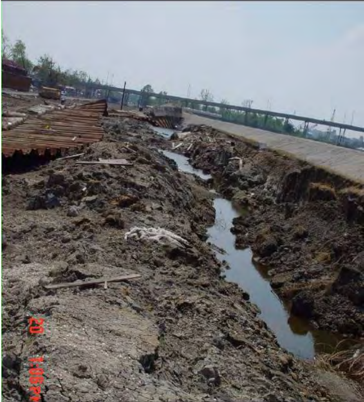
Figure 46. Scour and Erosion Leading to the Failure of the I-Wall on the IHNC Adjacent the South Breach (9th Ward)
