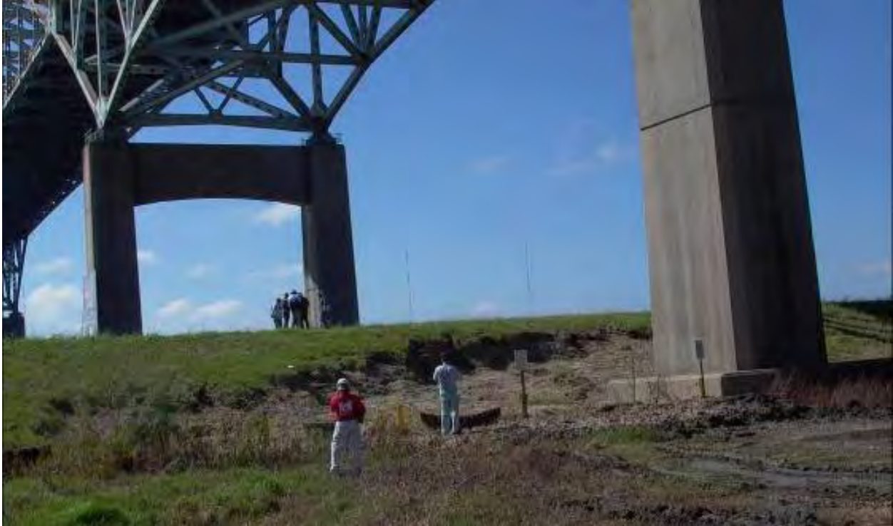
Figure 61. Overtopped Levee Under the Paris Road Bridge Adjacent to the Entergy Power Plant in the New Orleans East, After the Storm
