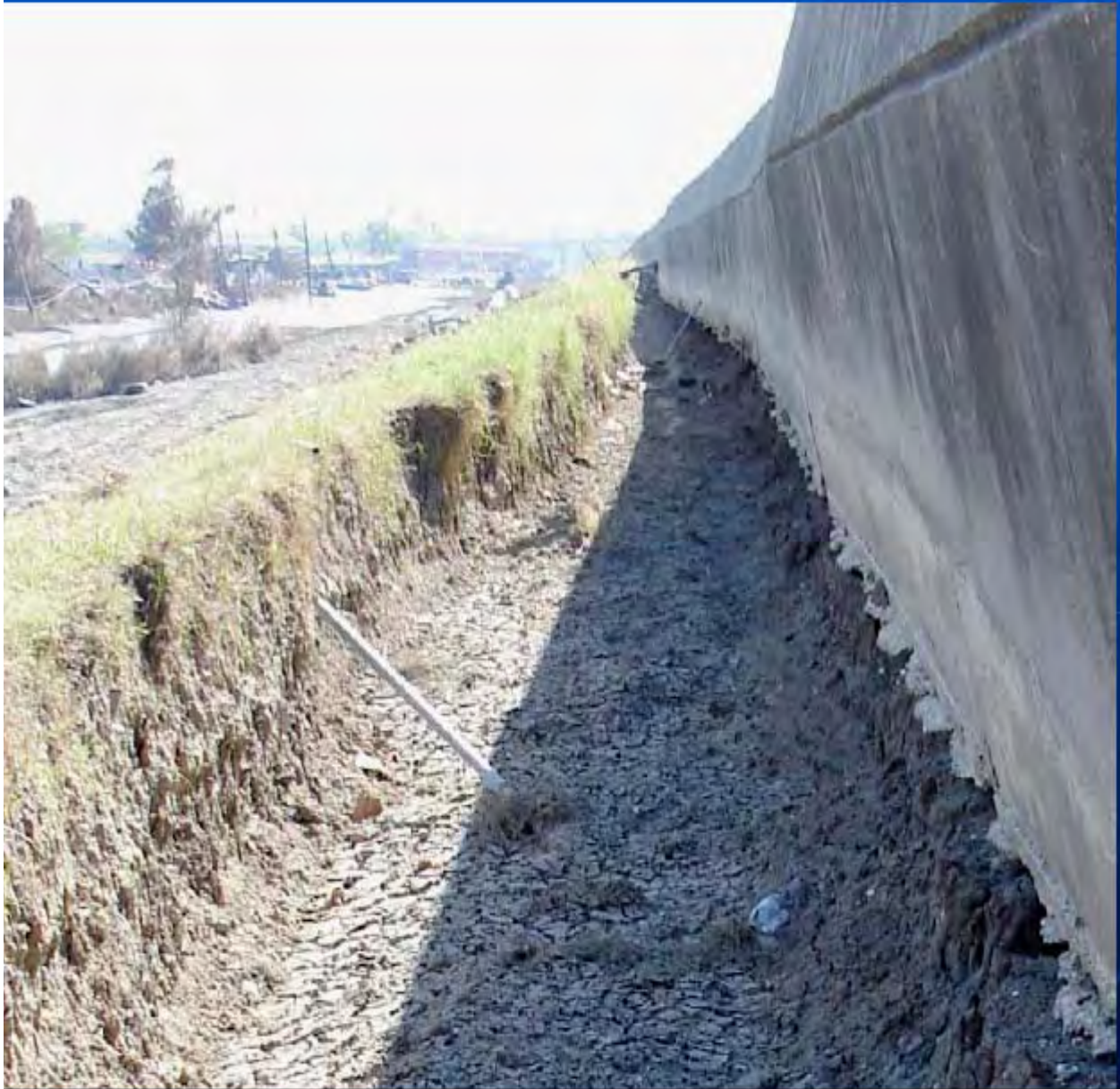
Figure 45. Scour and Erosion on the Protected Side of the IHNC Adjacent to the 9th Ward in the Vicinity of the South Breach
