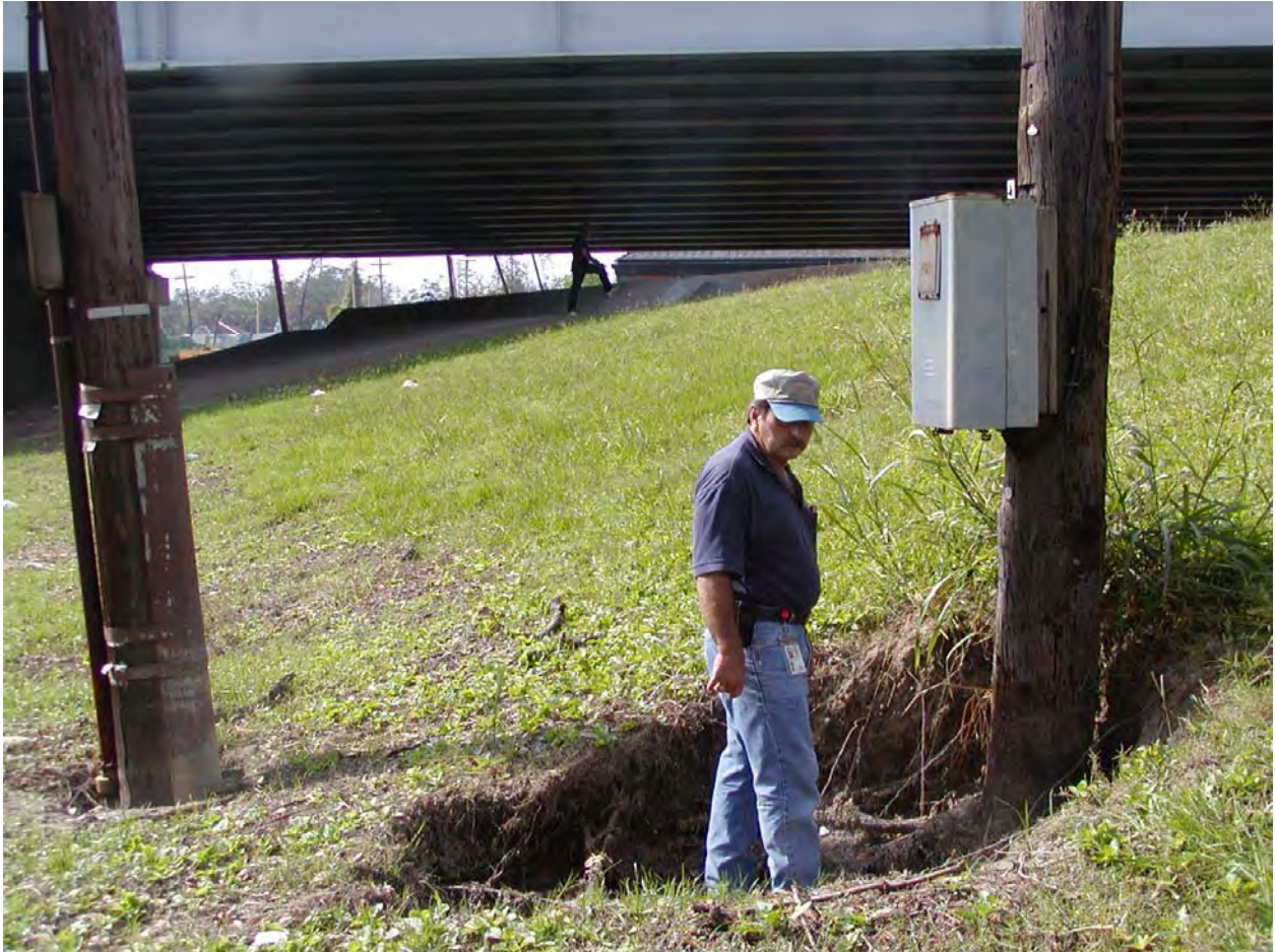
Figure 1-76. Scour around power pole below earth levee on east side of Orleans Ave Canal.
