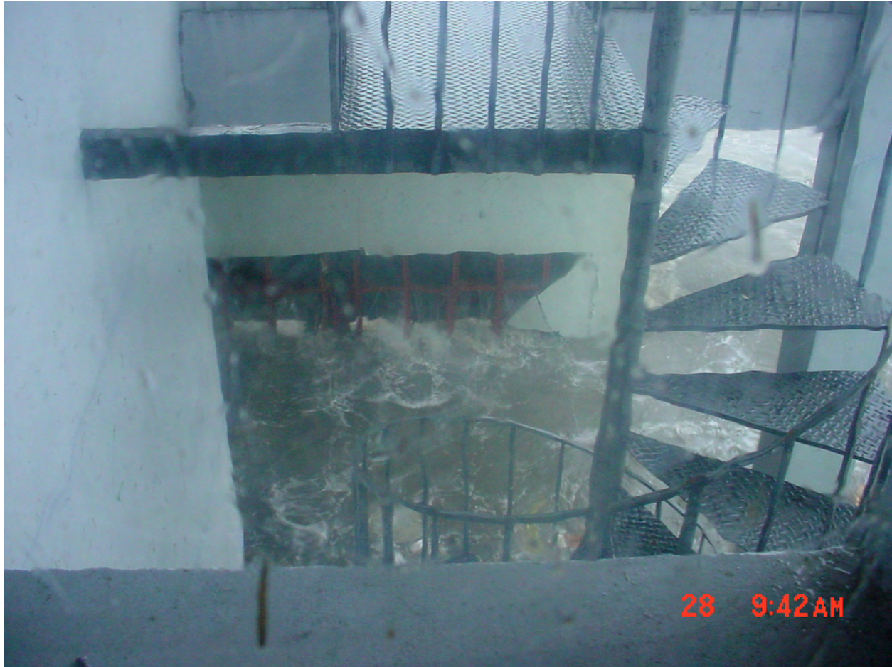
Figure 1-39. Time = 9:42 AM, APH-03. Wall north of east spiral staircase.
