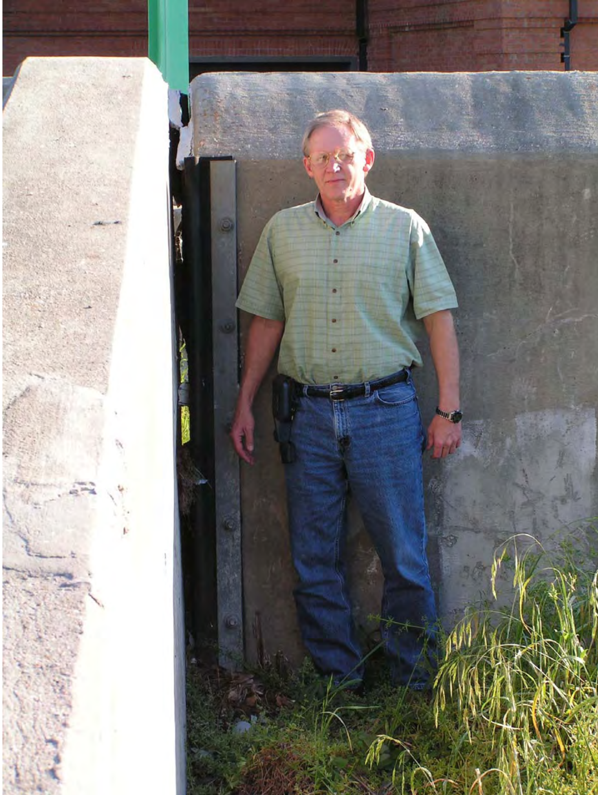
Figure 1-86. LA 1251 at crack in wall. Picture taken 4/06/06. Debris in crack was 2.2 ft below top of wall on 9/29/05.
