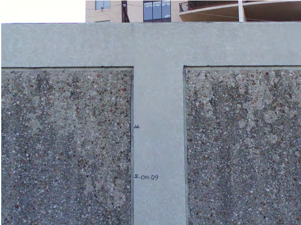
Figure 1-30. Time 11:00 on 8/29/05, elevation 12.5 ft (top of floodwall), 10.2 ft (peak of 2 ft waves), 9.2 ft (average water level at OM-09)
