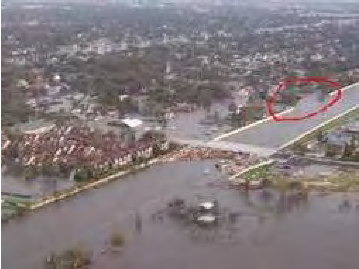
Figure 10-1. 17th Street Canal August 29, 2005. Looking south showing breach and debris impounded against Hammond Highway Bridge
