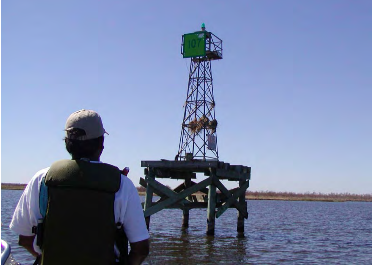
Figure 1-102. LA 1155 on MRGO. Debris on tower.
