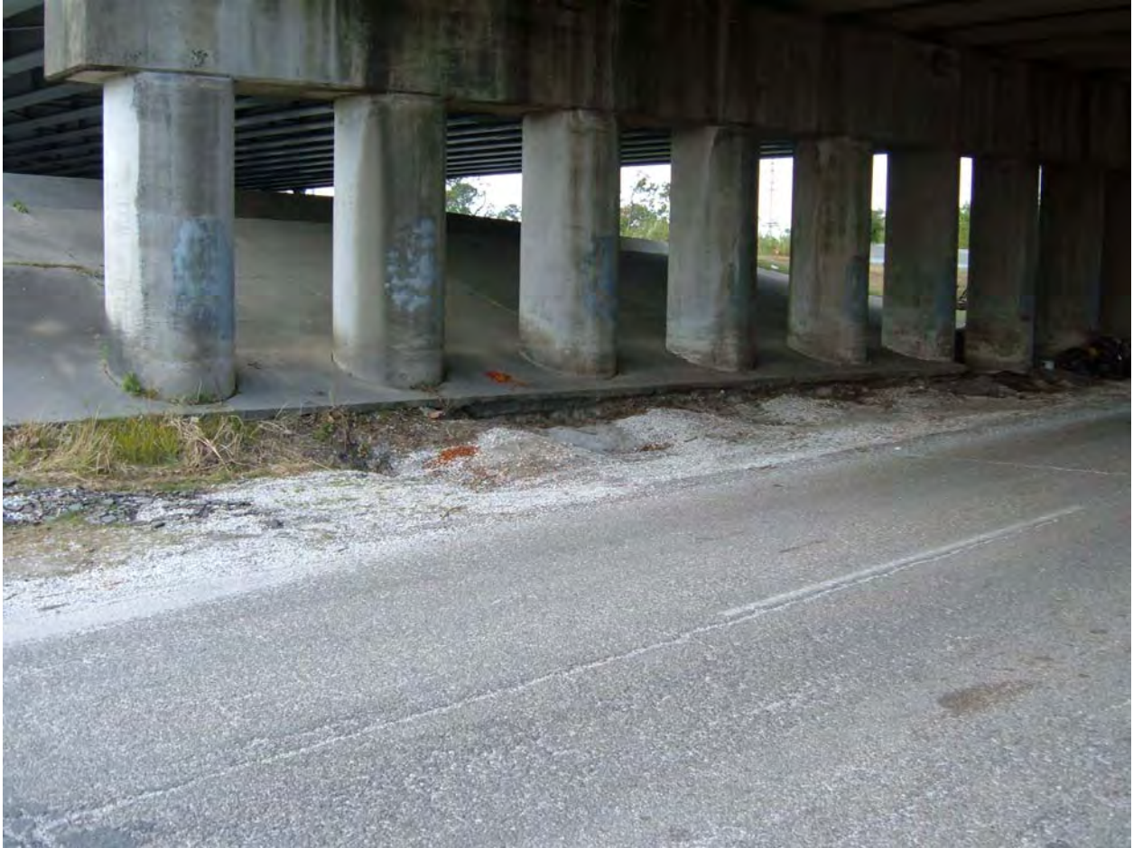
Figure 1-75. Scour between columns below low pump station wall at OP#7. Low wall is at top of slope behind concrete columns.
