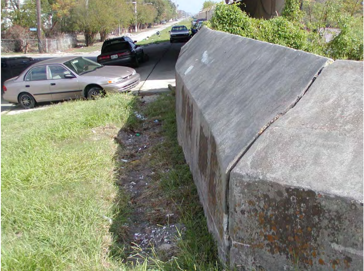
Figure 1-78. Scour below OP#7 low pump station wall on west side. Note that fall distance and scour is greater on this side than on the east side. Note floodwall in background that is about 4.3 ft higher.
