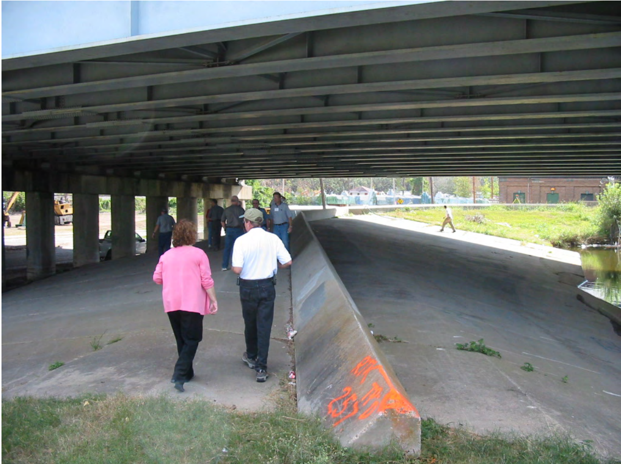
Figure 1-73. Low wall that connects to OP#7 at Orleans Avenue Canal looking south-southeast standing on earth levee.
