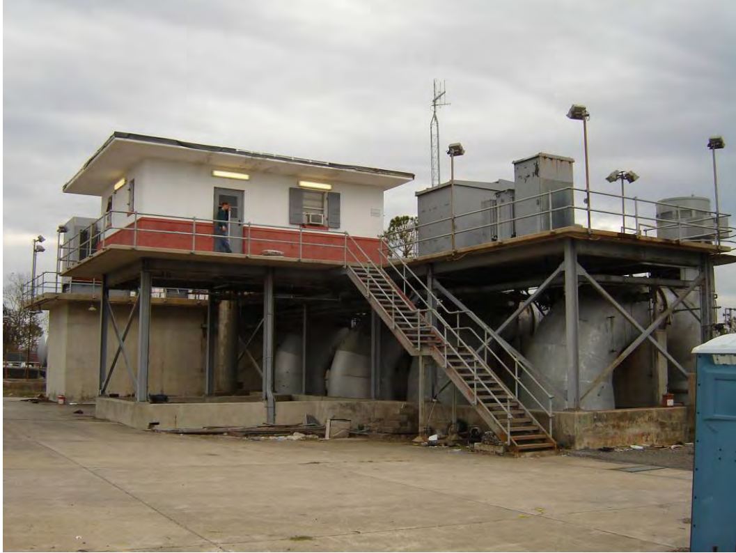
OP #16 -- ST. CHARLES PUMP STATION
