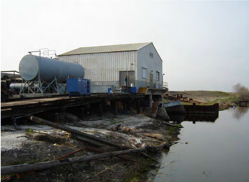
HAYES PUMP STATION
