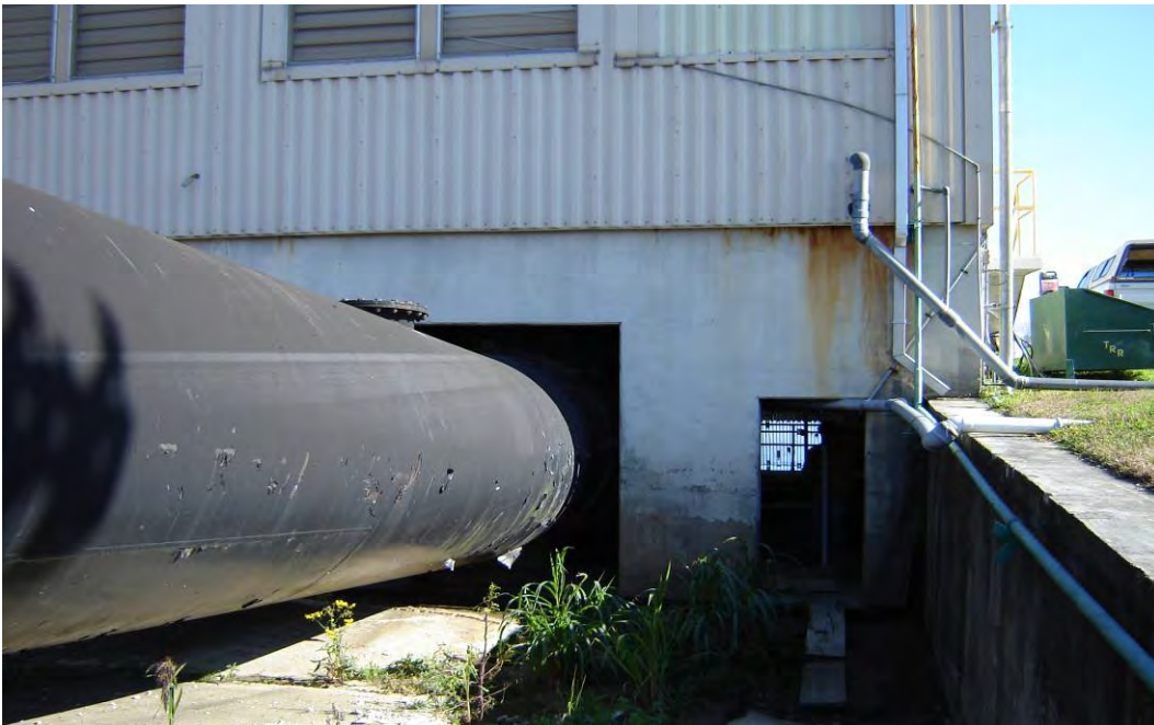
Ames Pump Station
