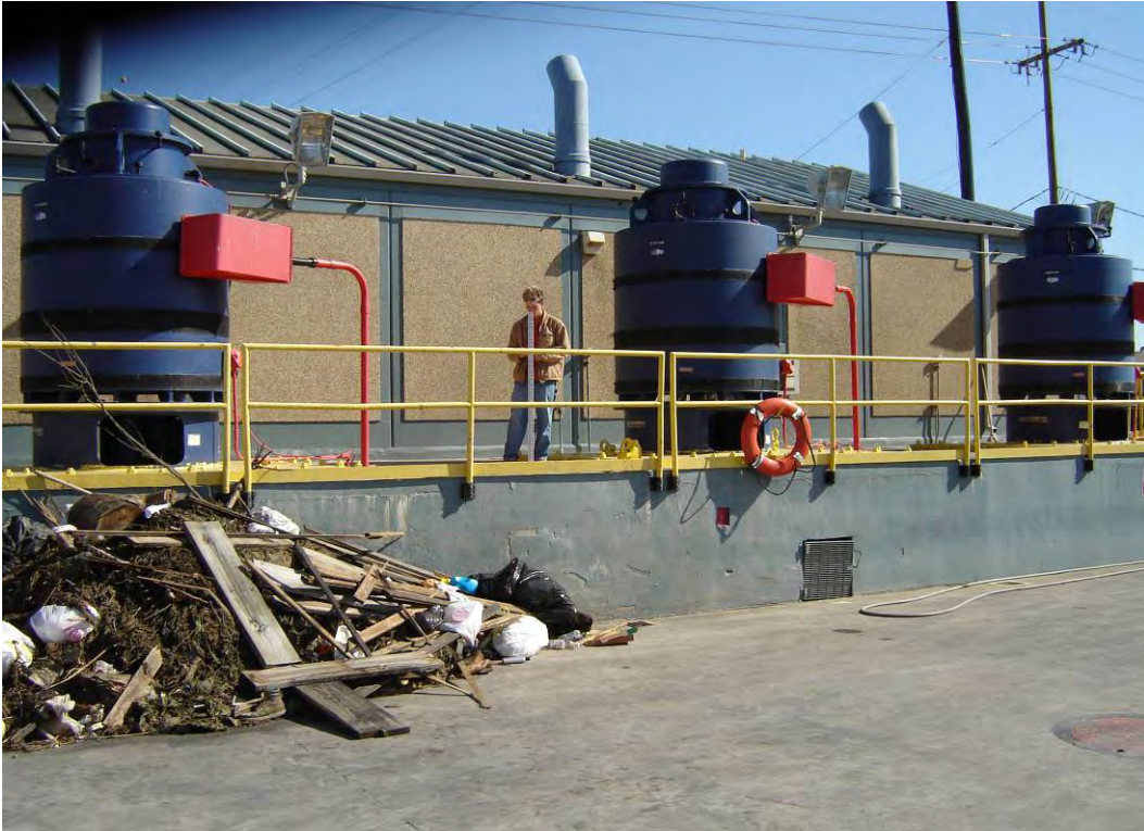
Harvey Pump Station
