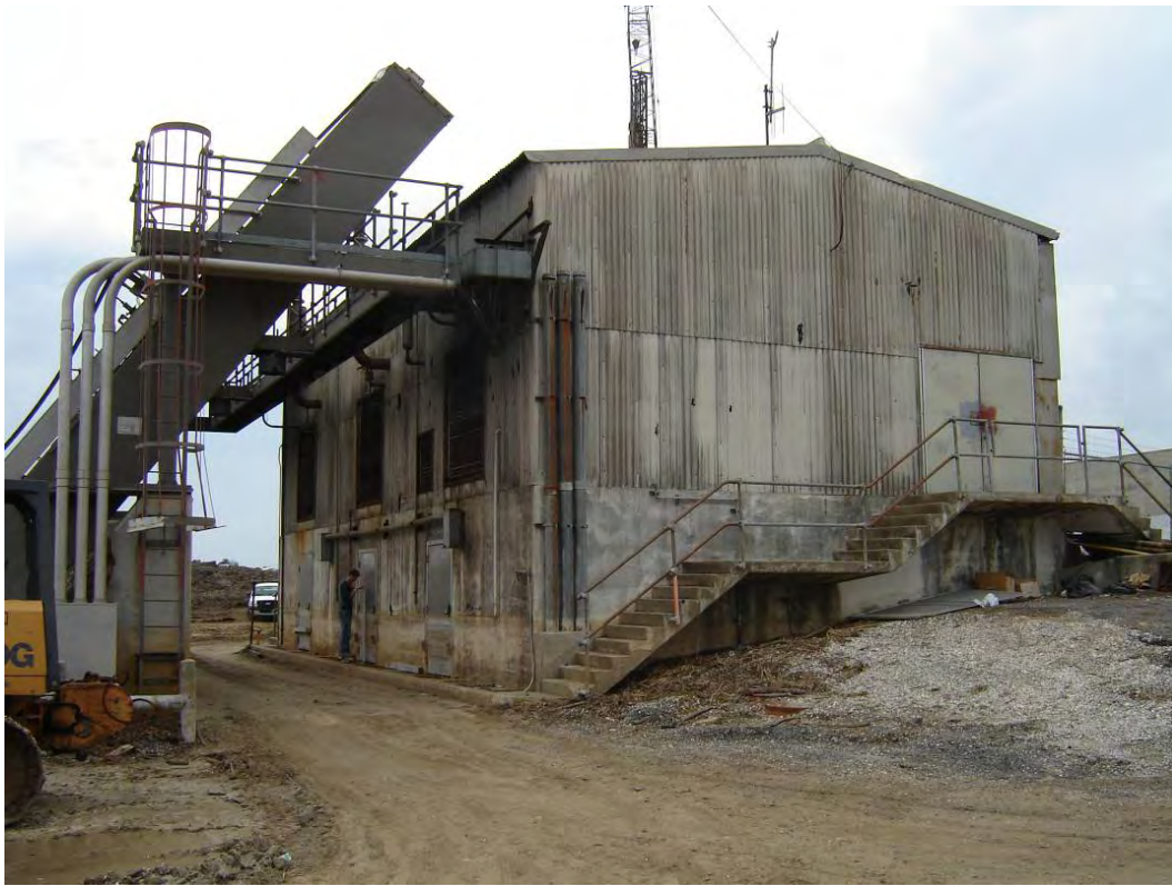
OP 15 Pump Station
