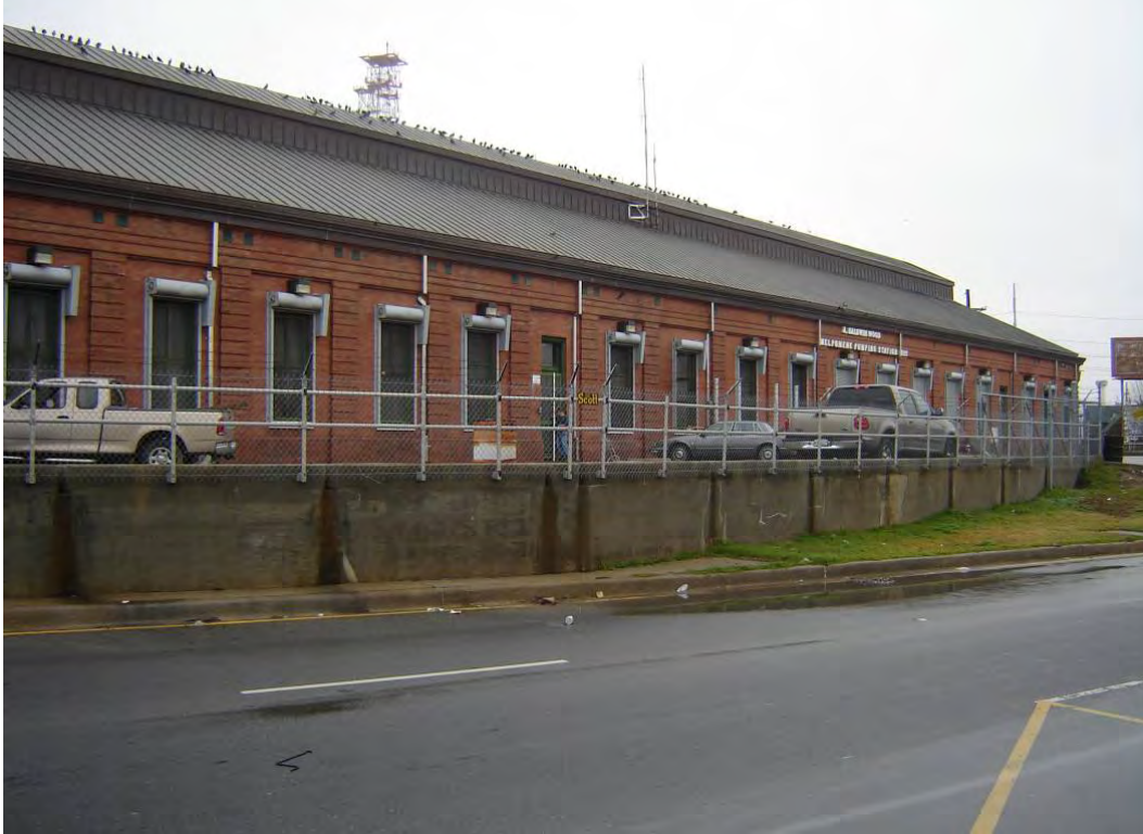
OP #1 Pump Station
