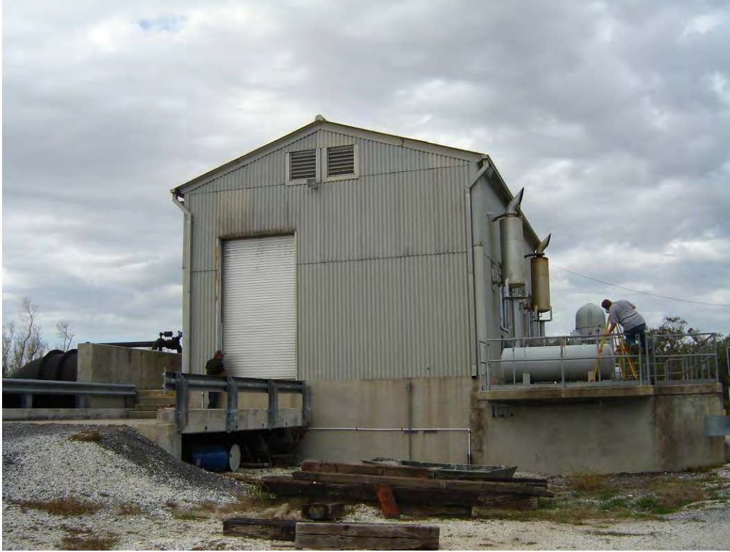
OLLIE #2 PUMP STATION
