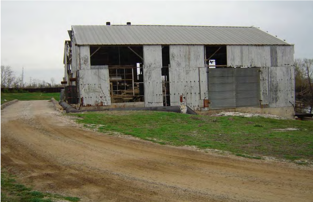
Guichard Pump Station #2
