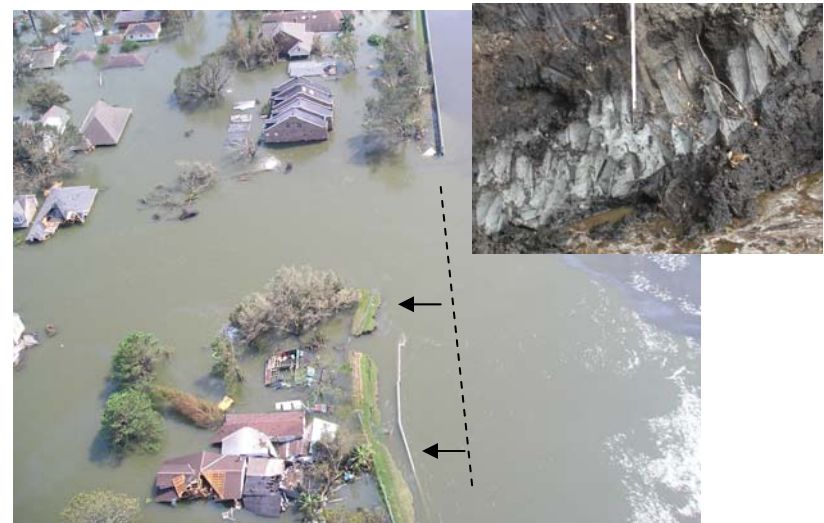
Displacement of wall and part of levee
