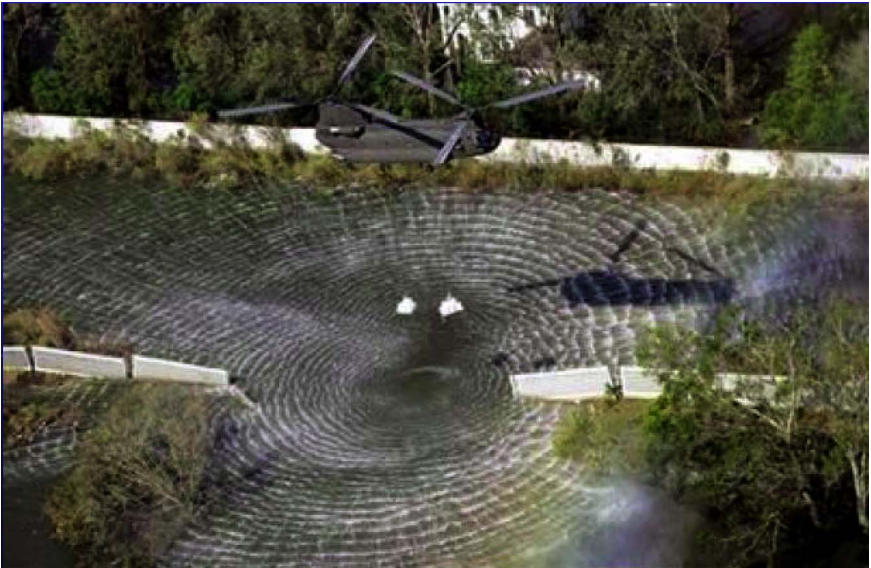
London Avenue south breach – about 60 ft wide – much sand washed through the breach into the neighborhood
