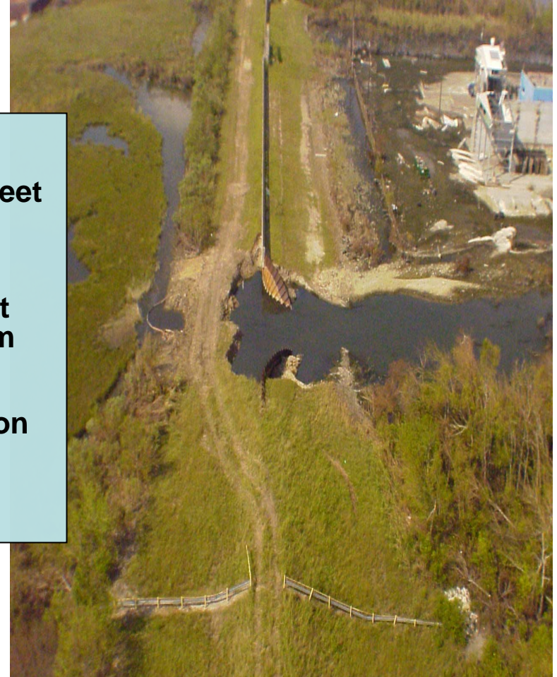
Figure 9. Floodwall Failure at East End of Michoud Canal FW
