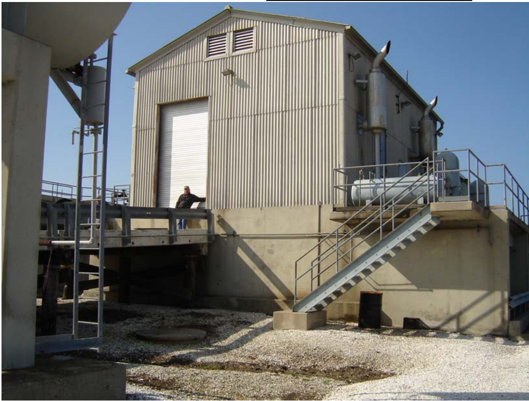
SUNRISE #2 PUMP STATION
