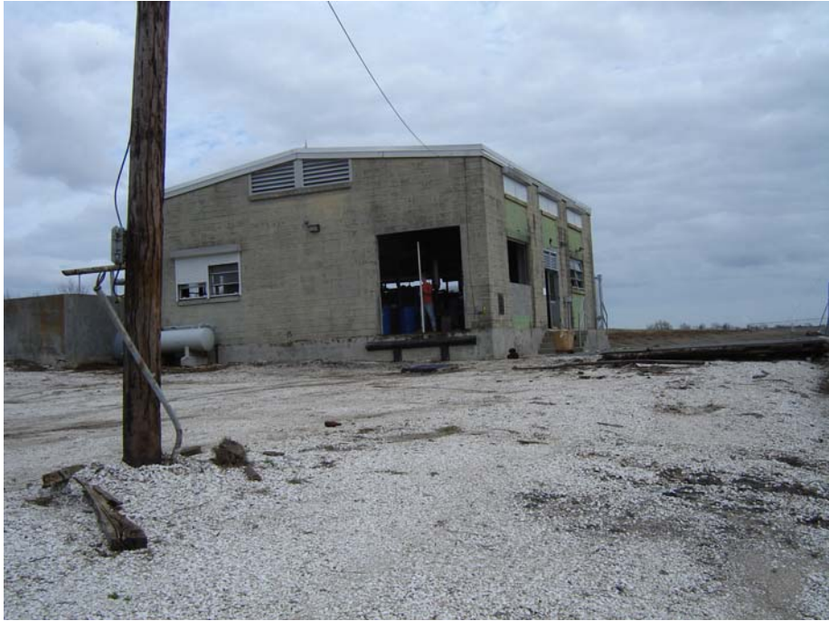
POINTE A La HACHE EAST PUMP STATION
