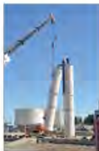
Crane removing first of two air stripper towers, used to treat contaminated groundwater at the former Castle AFB in Atwater, CA
