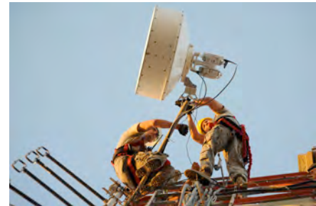
Perched on a 140-foot-tall communications tower adjusting a microwave antenna needed for network access
