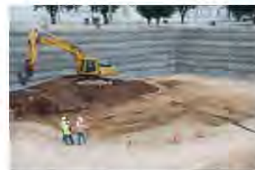
Soil excavation for water removal from a remediation site at former Kelly AFB, TX; preparation for a carbon source placement
