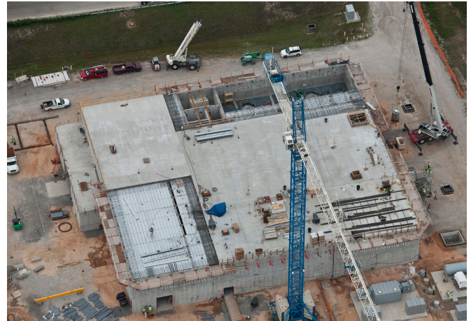
The WSB will process waste streams from the plutonium disposition process at SRS.
