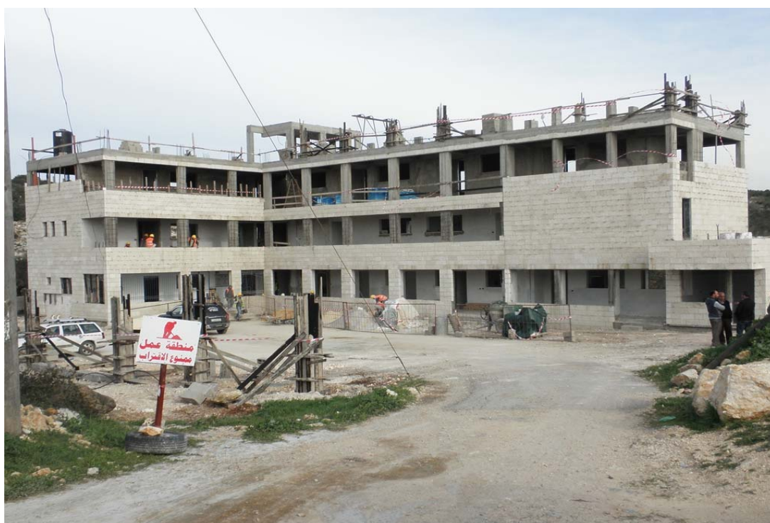
Workers construct Daher Al Abed School as part of a USAID-funded project. (Photo from CHF)
