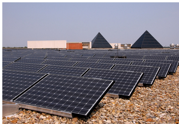
Figure 8. Solar PV installation at the Dallas VAMC.
