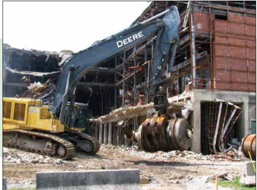
As part of the K-25 Building east wing demolition, a converter is being removed from the building and staged for shipment.
