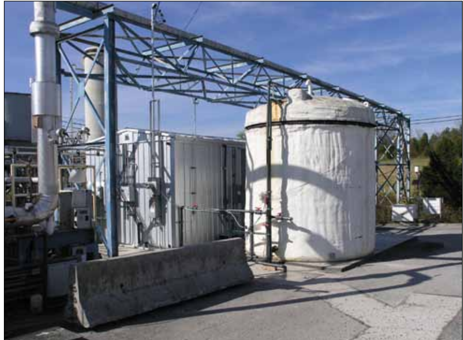
Chromium Water Treatment System
