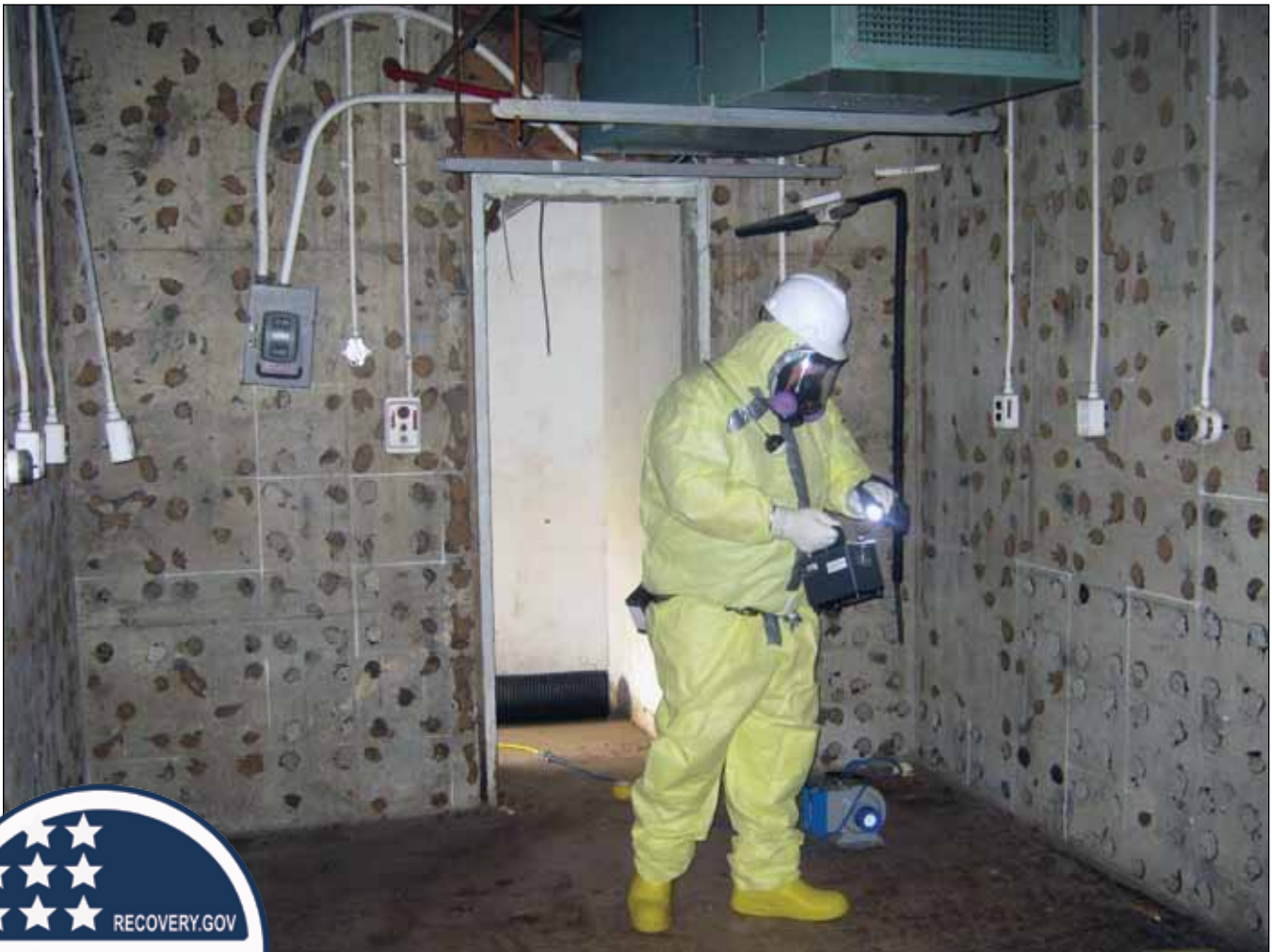
A worker conducts the final status survey inside the 3026 counting room, which is now ready for demolition.
