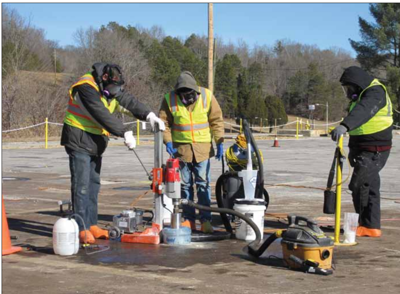
Workers sample the 2000 area slab, one of the selected areas where slab removal will be conducted as part of the Bethel Valley Soils and Sediment Project.
