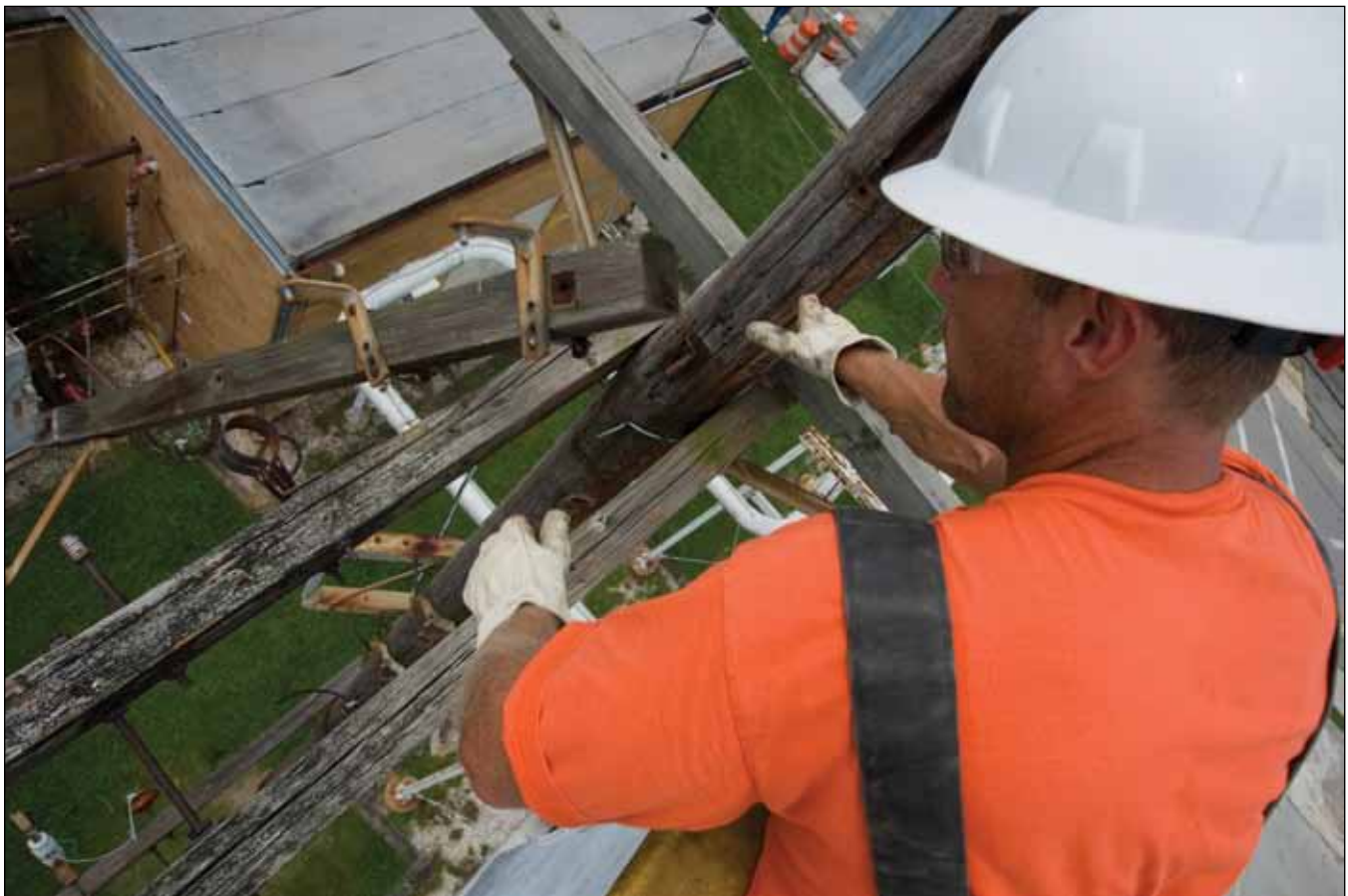
A worker dismantles infrastructure associated with Building 9735 as part of the demolition project.
