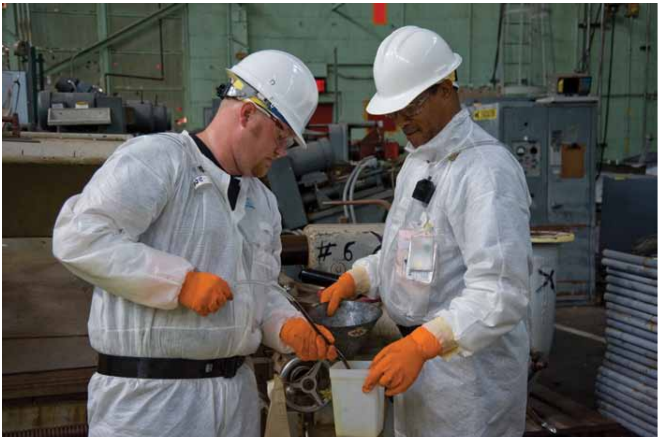
Workers are draining oil from legacy processing equipment in the Beta 4 facility.
