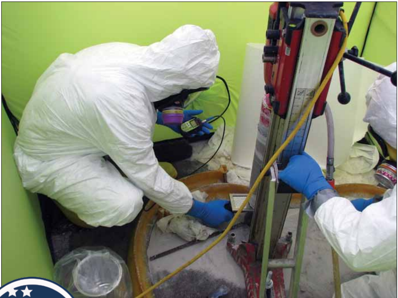
Workers perform underground duct sampling as part of the 4500 Gaseous Waste System Upgrades Project
