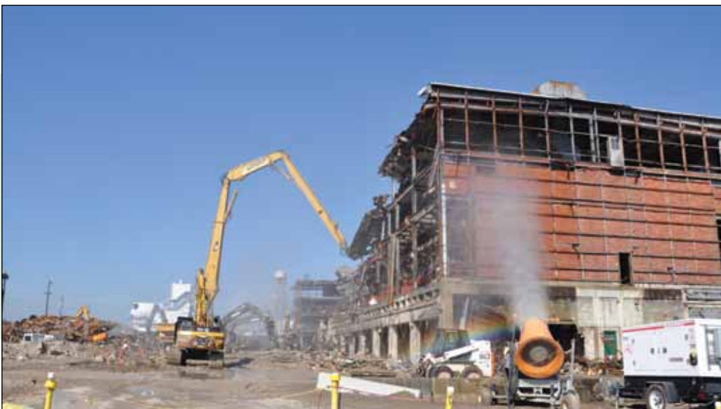
Misters spray water over the demolition area to help prevent dust from flying up while the building is being demolished.
