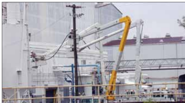
Upgrading and transferring ETTP's electrical distribution system to the City of Oak Ridge marked a major Reindustrialization accomplishment
