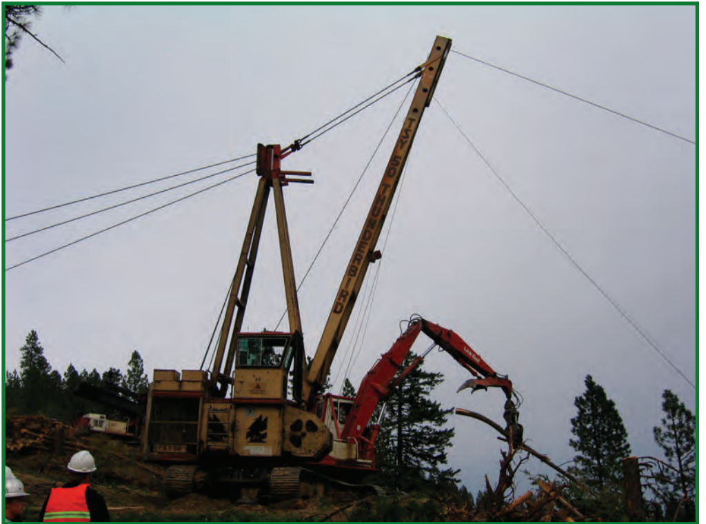
Figure 8.15. Yarder extracting whole trees or processed logs on steep ground (>35 percent slope).
