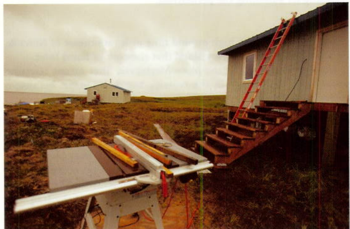
Three homes built at Mertarvik in 2006 are still being worked on. They may be moved.
