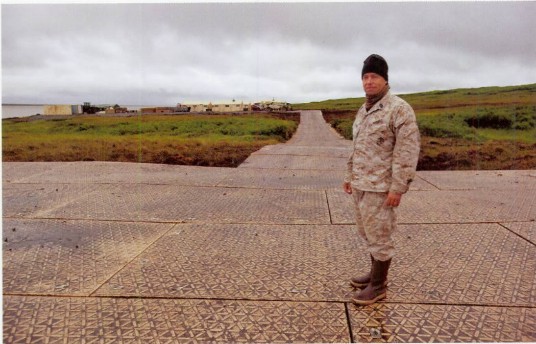
Master Sgt. Graham Hilson, camp commander, stands on top of the base for camp next year at Mertarvik. The current base will be used as a loading/unloading area.
