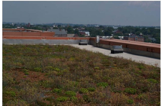
An extensive green roof on a Washington, D.C., office building (Source: C.E. Clark, Argonne National Laboratory)
