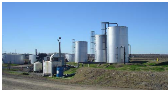
Tank battery used to separate and store oil and produced water.
