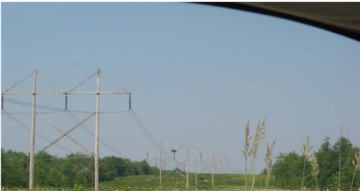
Existing 345-kV transmission line with Osprey Nest on Wooden H-Frame towers
