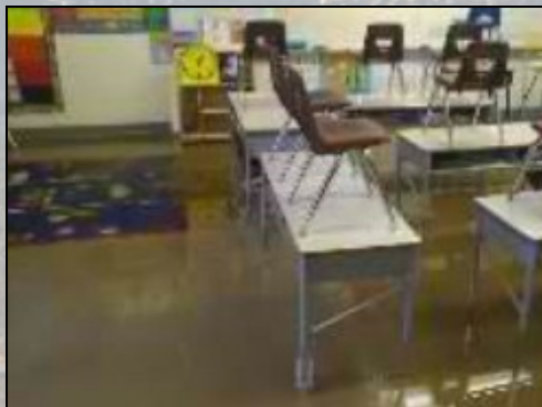
Flooded classroom at Saul Martinez Elementary due to a nearly stationary storm on September 11, 2012. (Source: KESQ TV)
