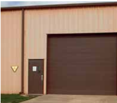
Mark contaminated buildings.
