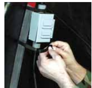
Don't overload receptacles.
