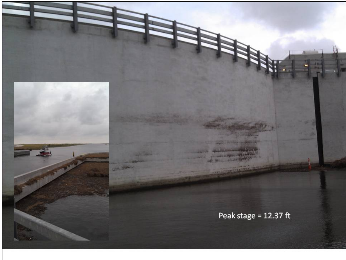
Figure 4.8 Damage assessment data from the IHNC Surge Barrier.
