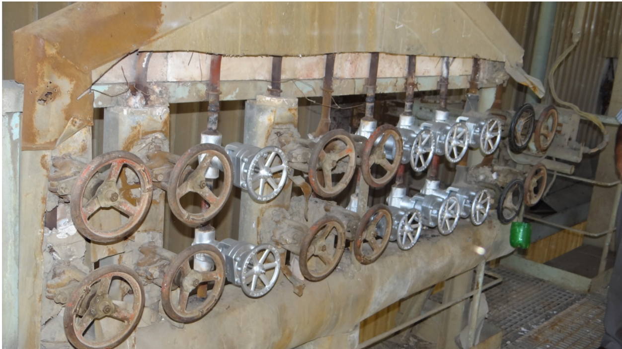
The project is replacing drain valves. The bright silver ones are new. (Photo by OIG, October 2012, Jamshoro)
