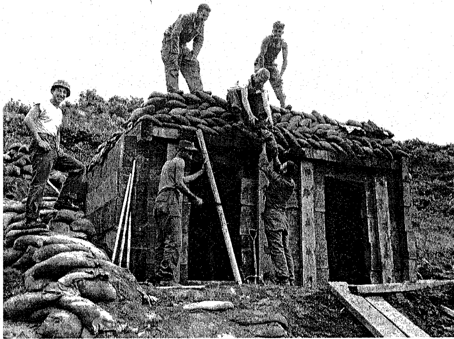
Precut Timber Bunker on Front Line, May 1953. The Troops Added Door Covers, and Floor Mats.
