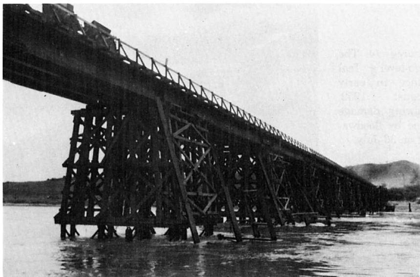
Figure 16. A survivor: the high-level Whitefront timber-pile bridge in September 1952 with damage largely limited to the fender piles.
