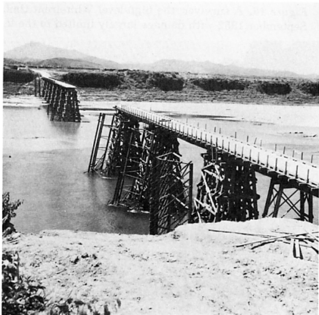
Figure 14. The high-level Teal bridge in early August 1952, showing damage done by floodwater on 30 July.
