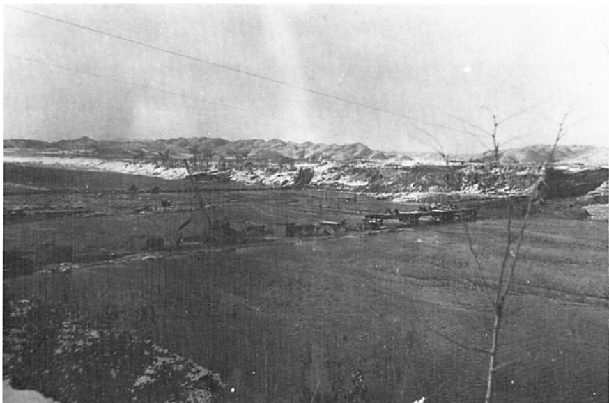
Figure 30. Girders in place on piers 8 through 11 allowing the passage of water below these spans and the construction of a causeway to pier 11 from the north bank.
