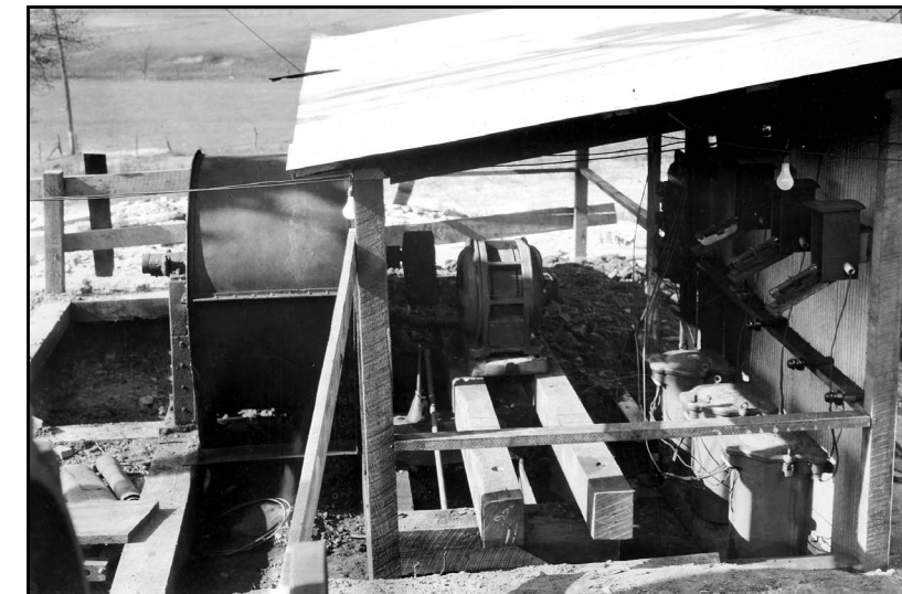
Sunday Creek Coal Company – Fan motors, transformers, and seal of the new air shaft. Photo Bureau of Mines
