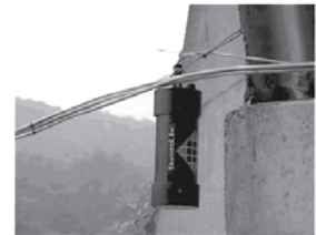
Radio Repeater At Portal
