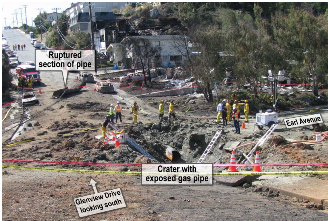
Figure 2. Picture of ejected pipe section.
