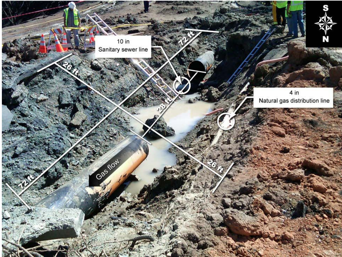
Figure 1. Picture of crater and ruptured pipeline.
