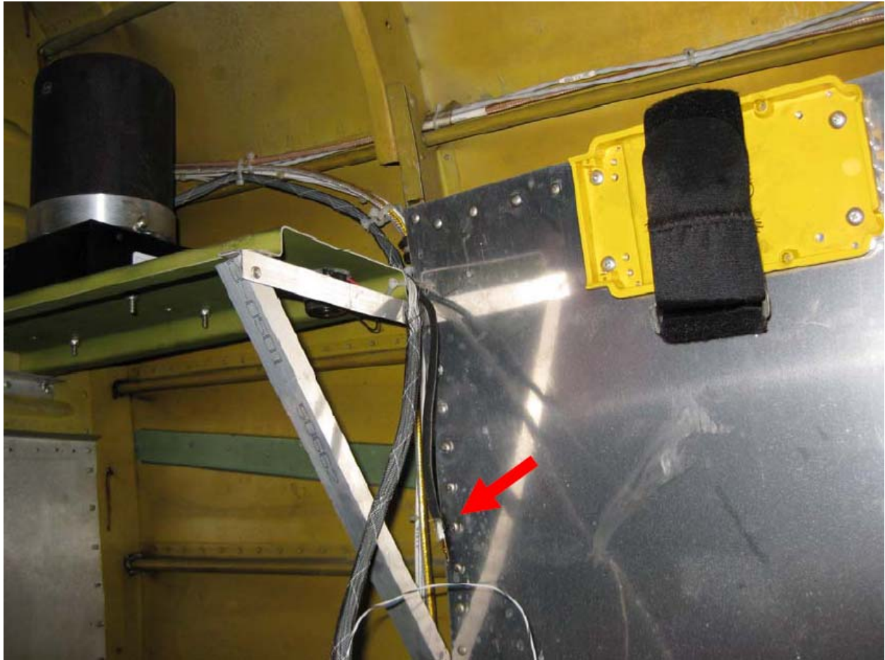
Figure 12. Accident airplane's emergency locator transmitter mounting tray and retention strap.
