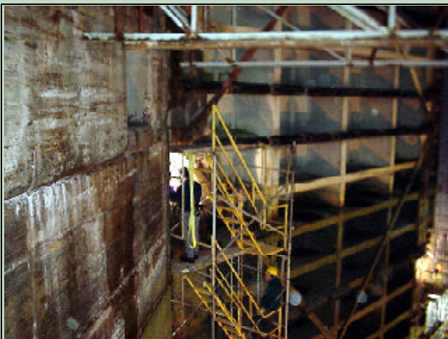
Workers are repairing cracks found on the downstream south miter gate leaf at Snell Lock.
