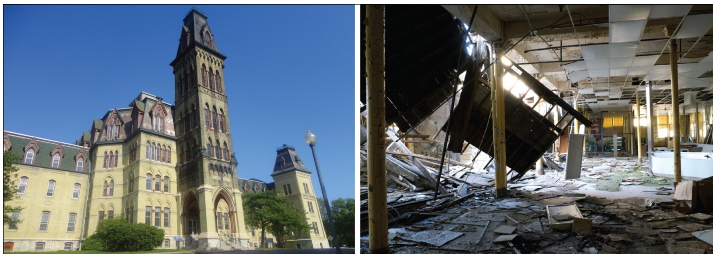
Figure 5: Deterioration of the “Old Main” Hospital, Built in 1869, at VA’s Medical Center in Milwaukee, Wisconsin
