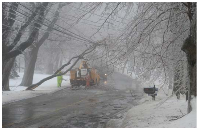
Figure 3. Road crew working on downed tree branches and wires near Burlington, Connecticut after ½” or more of ice fell on March 2, 2007 (Image courtesy of WFSB-TV Hartford, CT).
