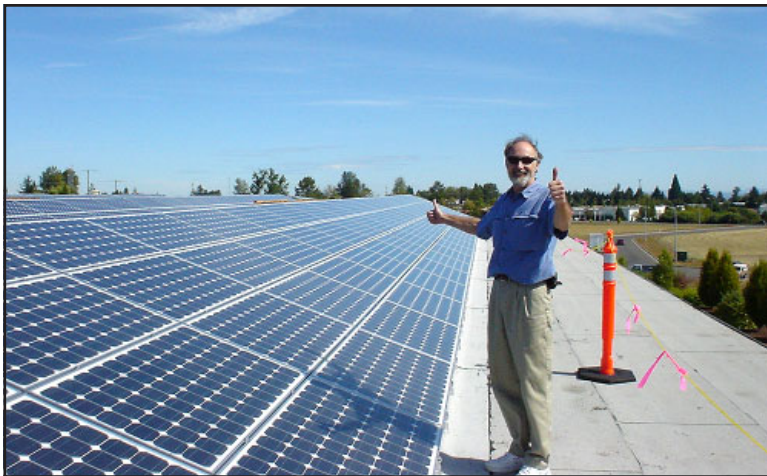
Figure 25 — Solar contractor David Parker gets thumbs up from Kettle Foods in Salem.
