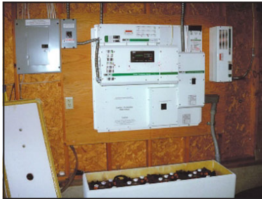
Figure 21 — Power panel with battery box
