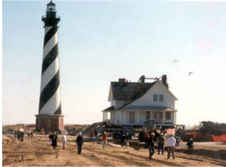
The principal lighthouse keeper’s quarters being moved at Cape Hatteras NS, in advance of the move of the lighthouse itself. Photo: NPS.
