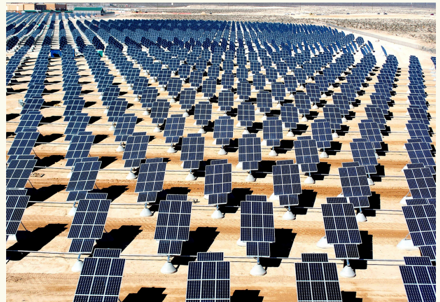
The solar photovoltaic array at Nellis Air Force Base.
