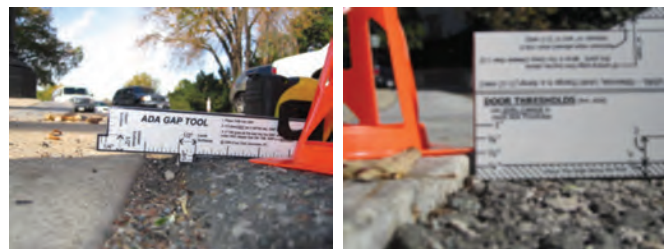
Slab Joint Too Wide & Too Deep Transition Too High
