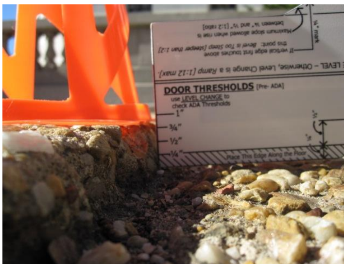
Example of Barrier Created by Level Change
