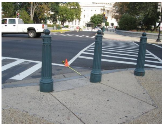
Ramp Outside of Marked Crosswalk (Curb Ramp 16)
