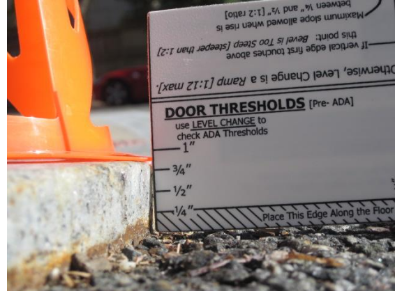
Transition Too High (Curb Ramp 27)
