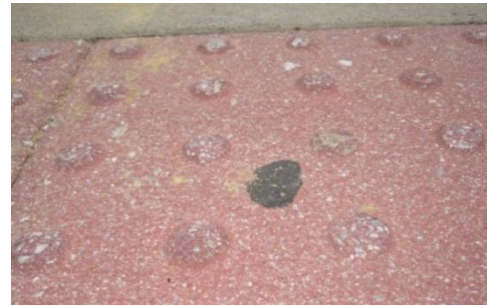
Deteriorated Detectable Warning (Curb Ramp 39)
