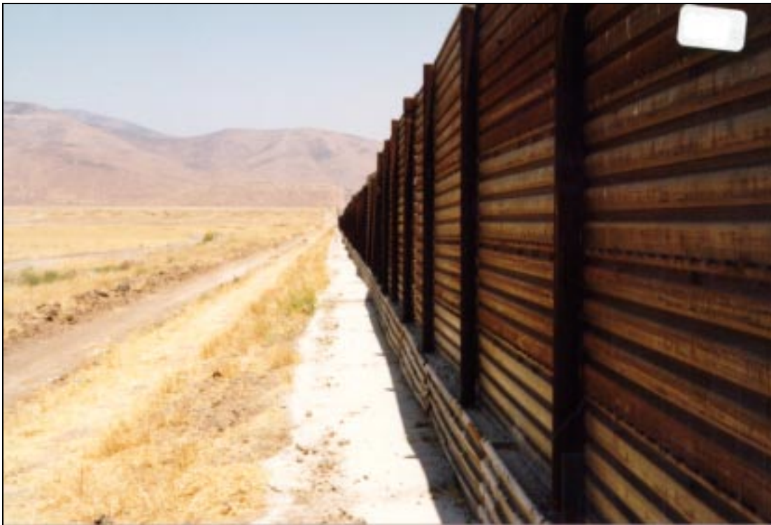
Figure B.23. Flat region of fence east of Otay truck entry point.
