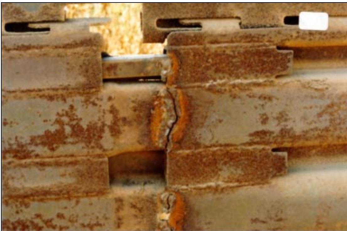
Figure B.13. Broken welds between mats and a repair made by welding one side of the square attachment pin.
