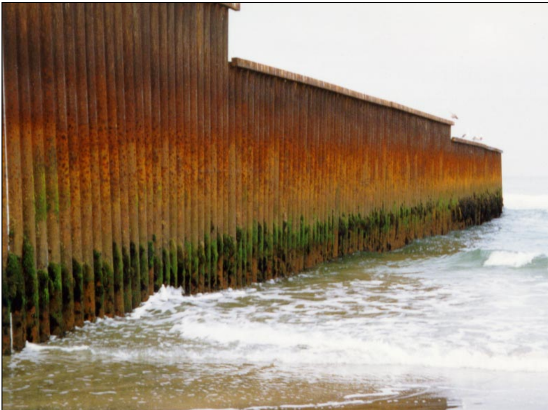
Figure B.1. Sea water corrosion on border fence.
