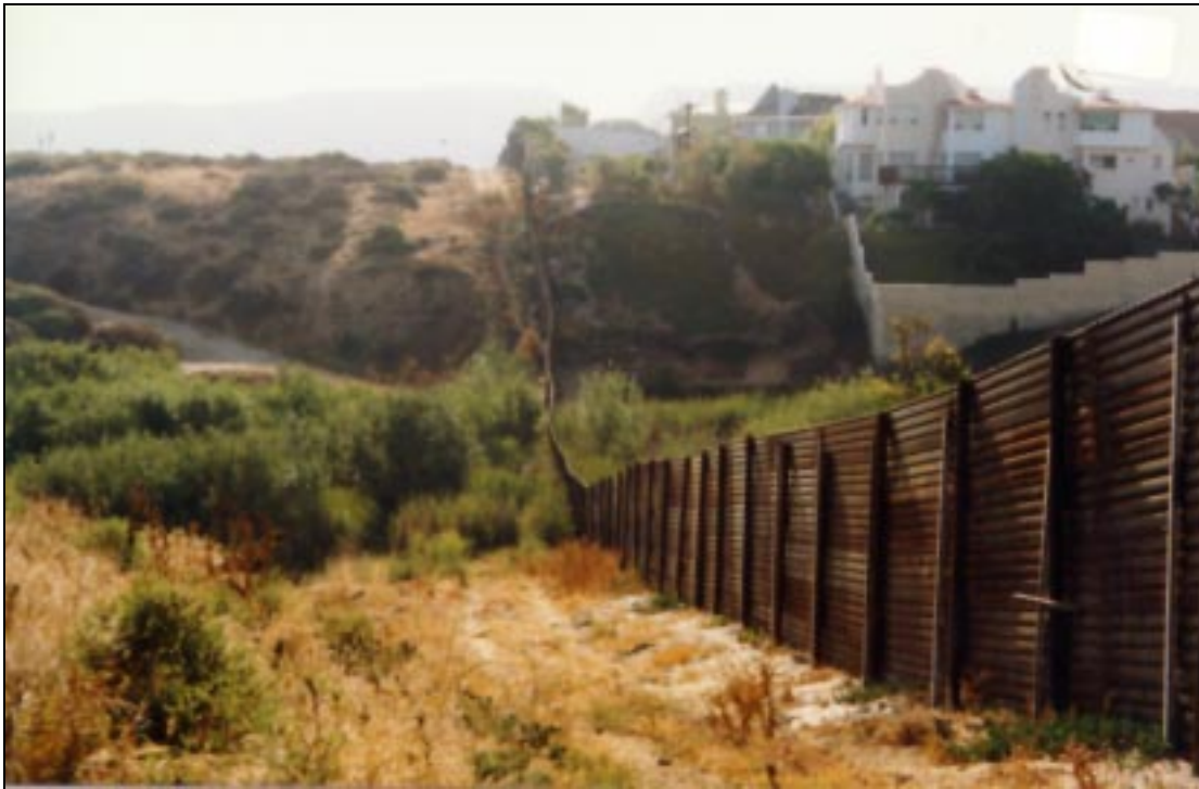
Figure B.7. Fence is bowed from thermal expansion as it extends inland.
