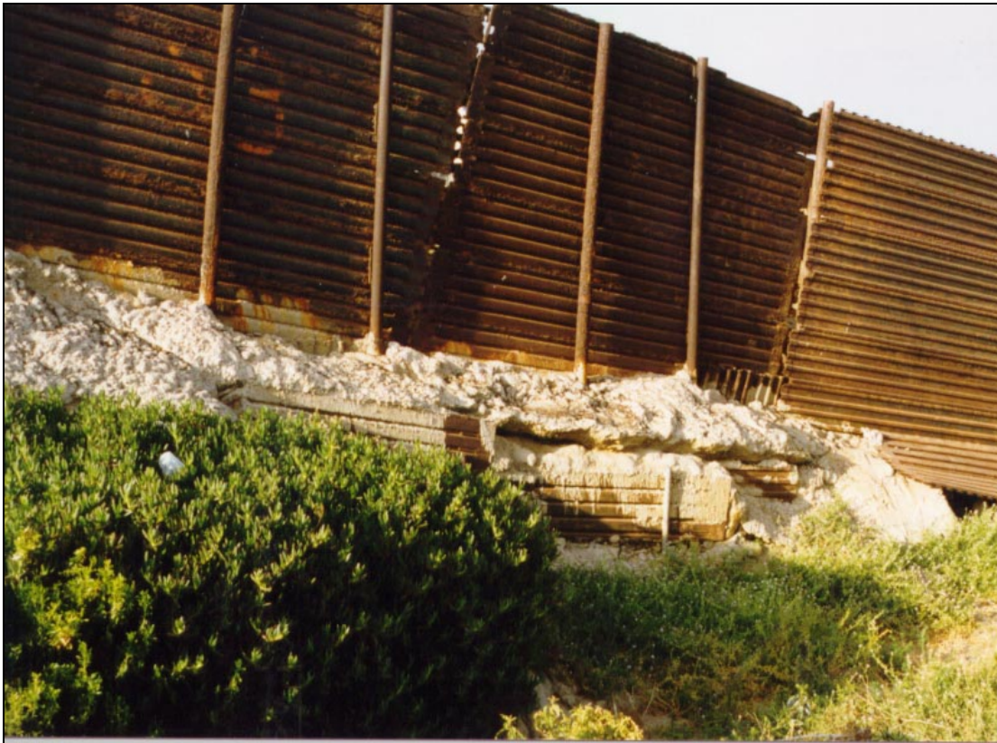
Figure B.4. Concrete poured into holes under the fence as a result of dig-under breaches and erosion of the loose beach sand.
