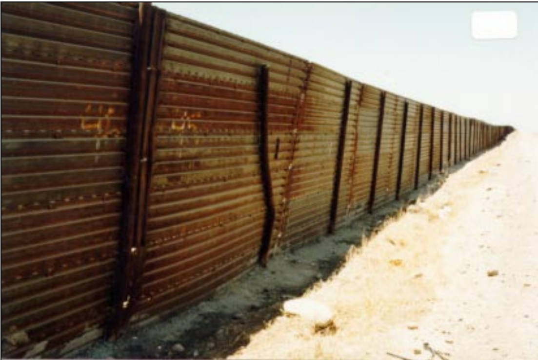
Figure B.21. Fence running between the hills and the Tijuana Airport is repaired from a truck collision on the Mexican side.
