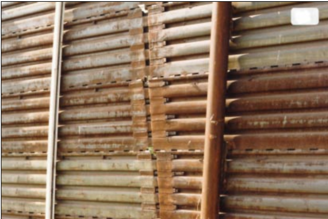
Figure B.8. Mats still have paint only 700 ft inland, and sections are connected by square pins and welded to vertical pipes.
