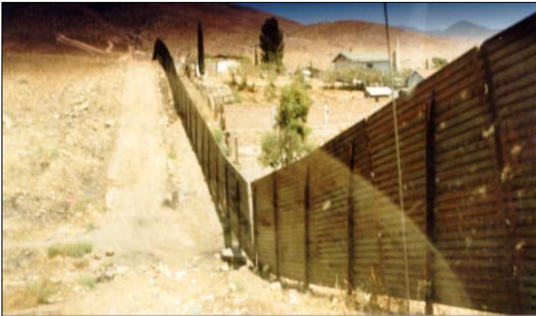
Figure B.27. Gaps exist under the fence, and a break in the section is seen at the bottom of the hill.
