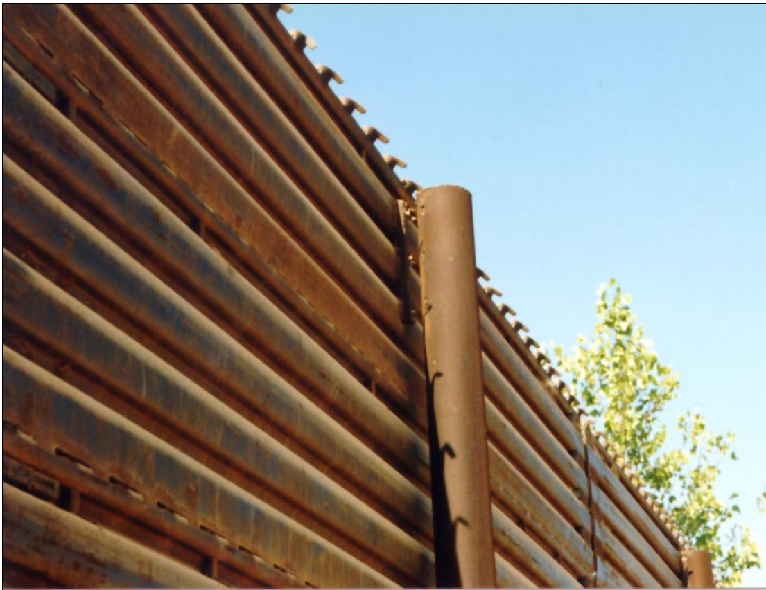
Figure B.12. Welds between the mat and poles are broken from thermal stresses.
