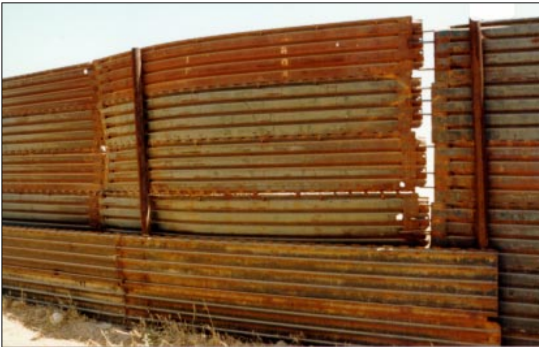
Figure B.25. This fence is still intact after being damaged by car ramming.
