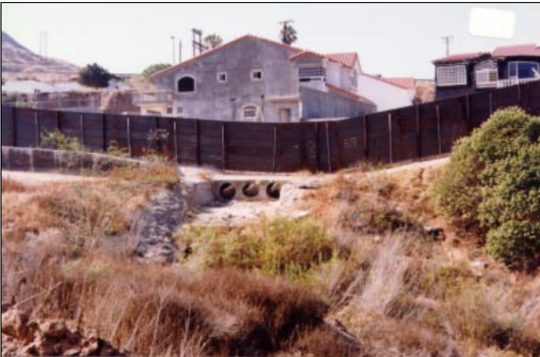
Figure B.10. The high traffic through the drainage tubes under the fence has buffed the metal interior to a shine.
