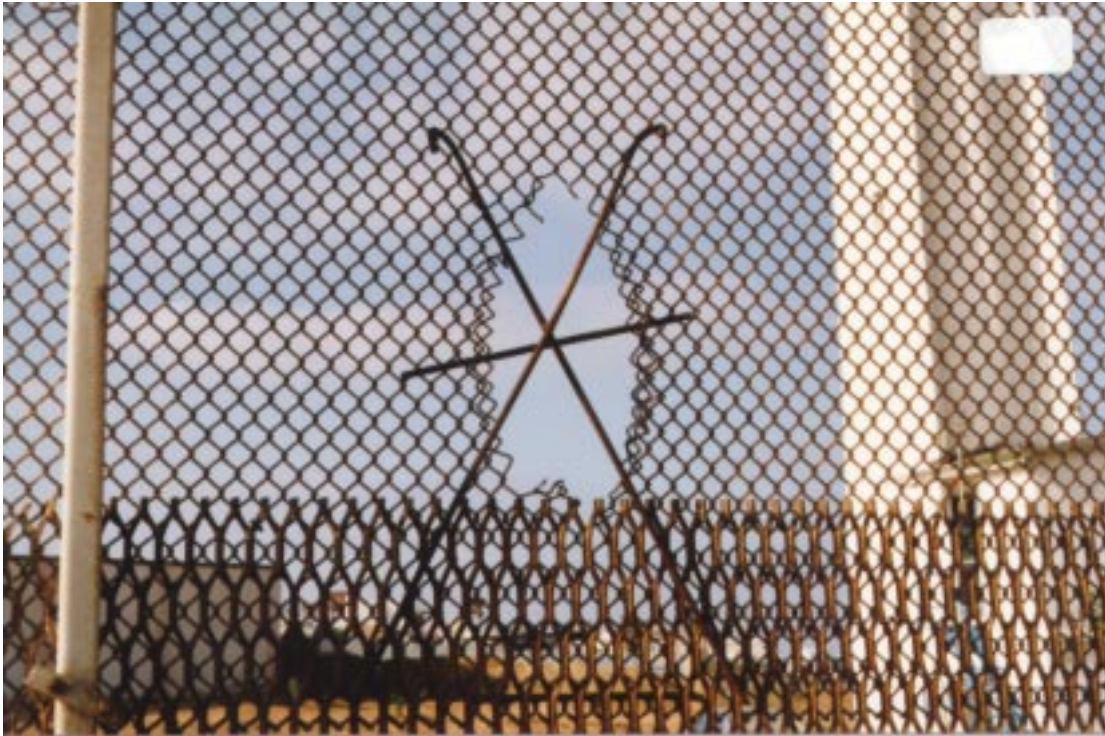
Figure B.6. Ad-hoc repairs to the chain link fence.
