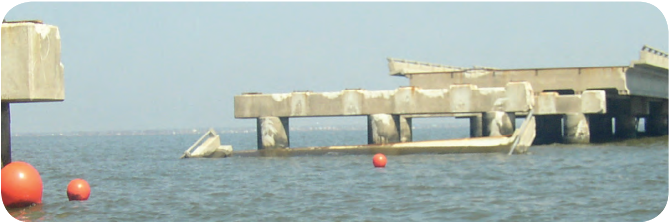
Figure 6. Westbound bridge of Interstate 10 Twin Span Bridge between New Orleans and Slidell, La., with collapsed and missing bent.
