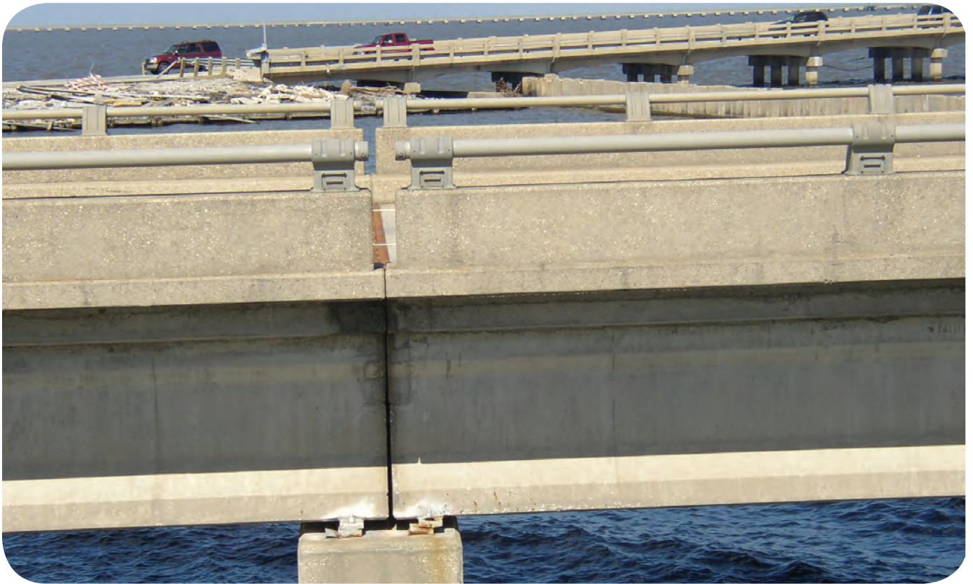
Figure 8. Close spatial proximity of Interstate 10 Twin Span Bridge (front), U.S. Highway 11 bridge (middle), and railroad bridge (back) across Lake Pontchartrain between New Orleans and Slidell, La.
