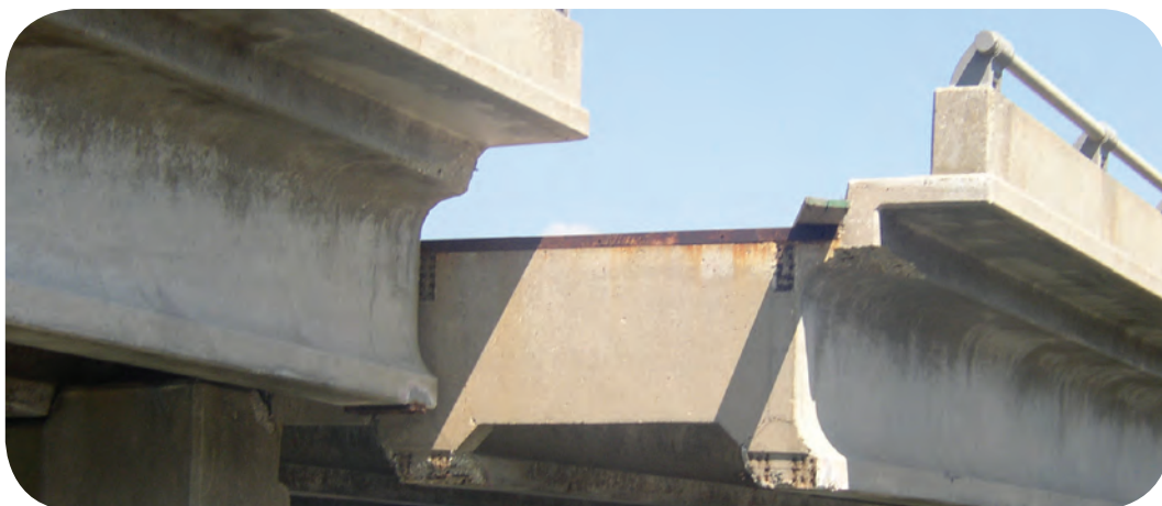
Figure 7. Westbound Interstate 10 Twin Span Bridge between New Orleans and Slidell, La., exhibiting excessive lateral displacement of approach's causeway deck. Decks stopped lateral displacement after a distance of one or two girder spacings.
