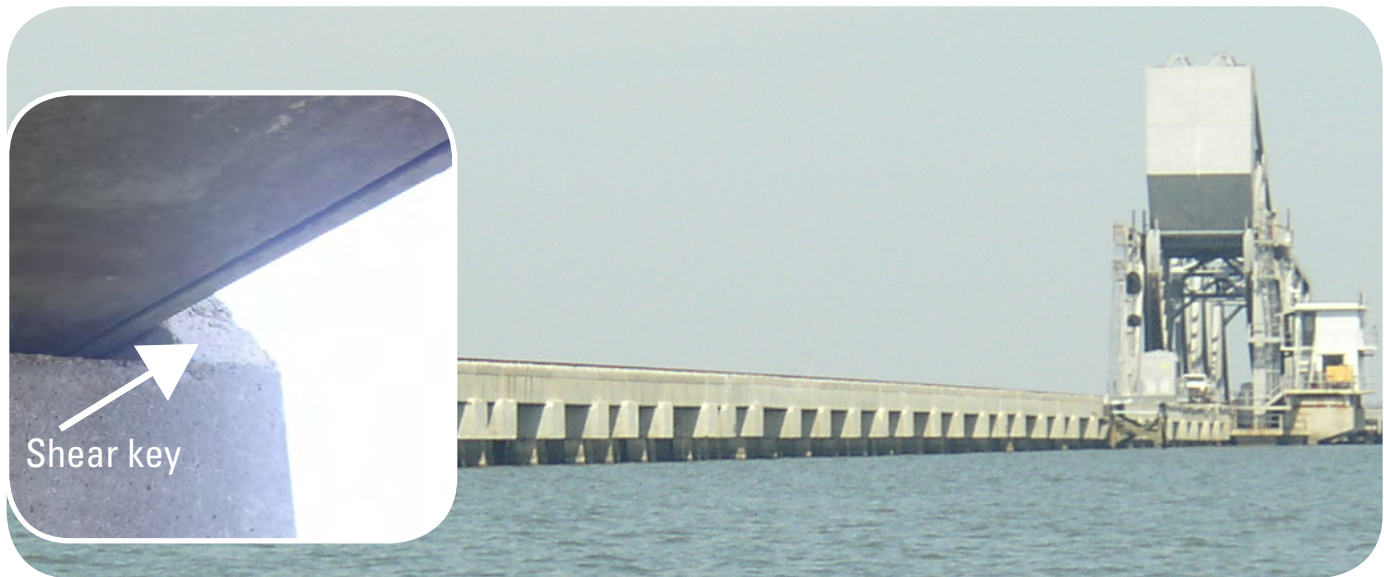
Figure 10. Overview and deck details of the railway bridge adjacent to Interstate 10 Twin Span Bridge between New Orleans and Slidell, La.; inset photo shows important differences such as the use of a solid deck (no hollow space underneath) and a shear key at ends of each cap beam (to prevent lateral movement).
