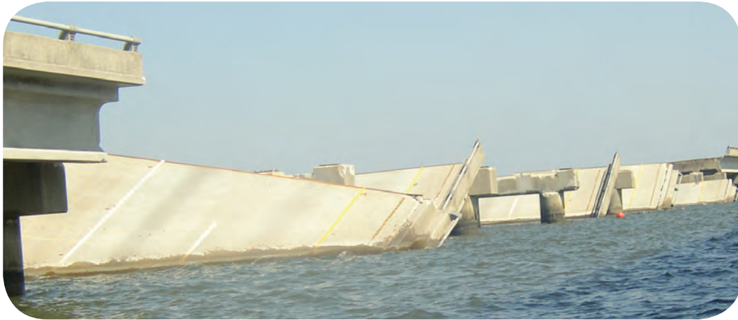
Figure 5. Interstate 10 Twin Span Bridge's causeway approach spans dropped off of bent cap beams. One end of each span is in the water.
