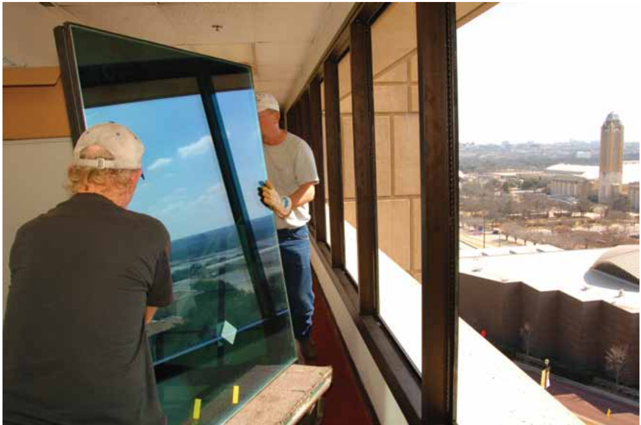
Workers install more energy efficient windows in the Education and Administration Building.
