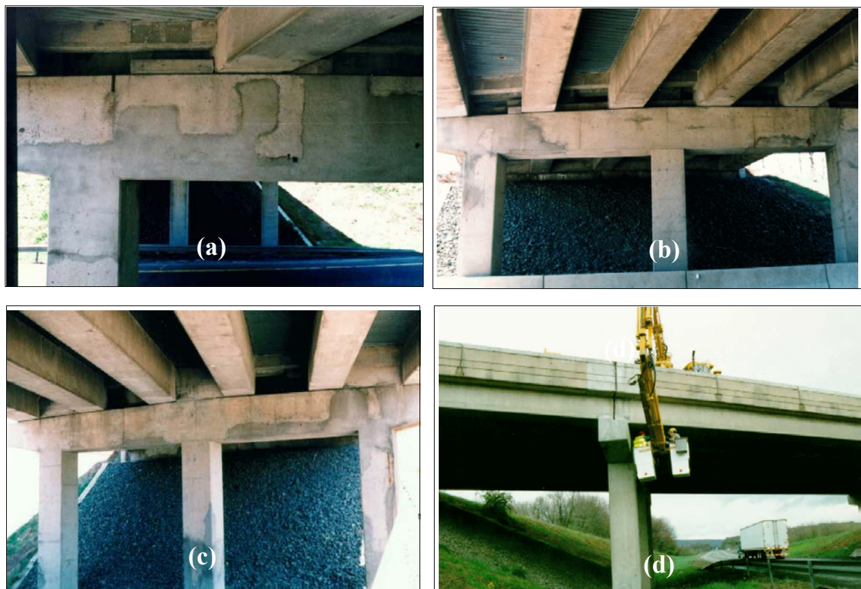
Figure 3-2. General views of piers: (a) pier 1, (b) pier 2, (c) pier 3, and (d) field evaluation in progress.
