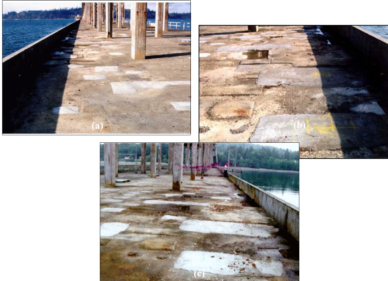
Figure 4-2. Partial views of test cells on the Hood Canal bridge: (a) cell 1D (control), (b) cell 2D (MCI 2020/2000), (c) cell 3D (Postrite/DCI).
