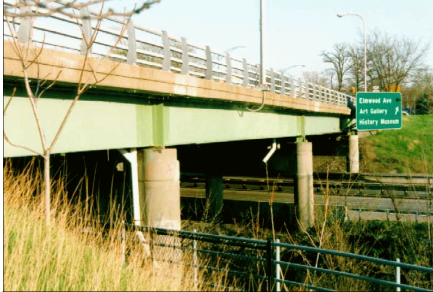
Figure 2-1. General view of the Elmwood Avenue bridge over NY Route 198, Buffalo, NY.
