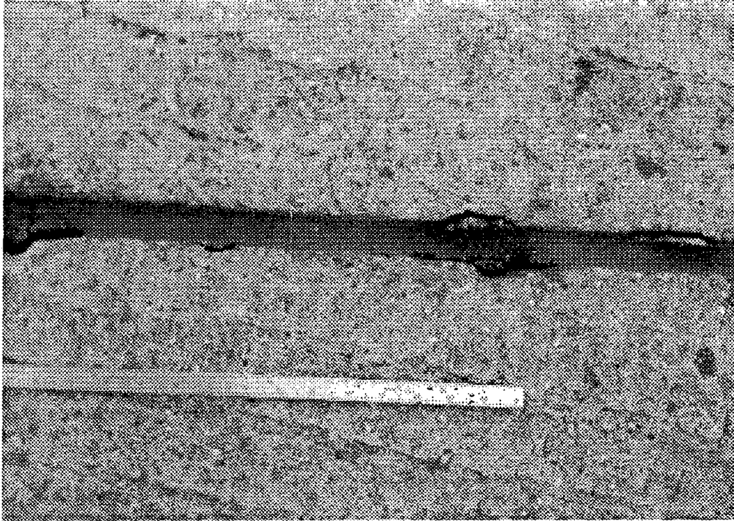
Figure 31. Spall failure in self-leveling silicone seal.
