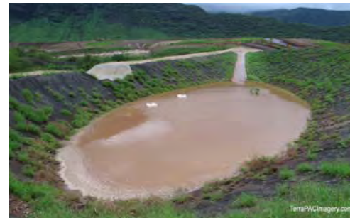
Newly constructed storm water retention pond at the PVT landfill in Nanakuli, Oahu, Hawai'i
