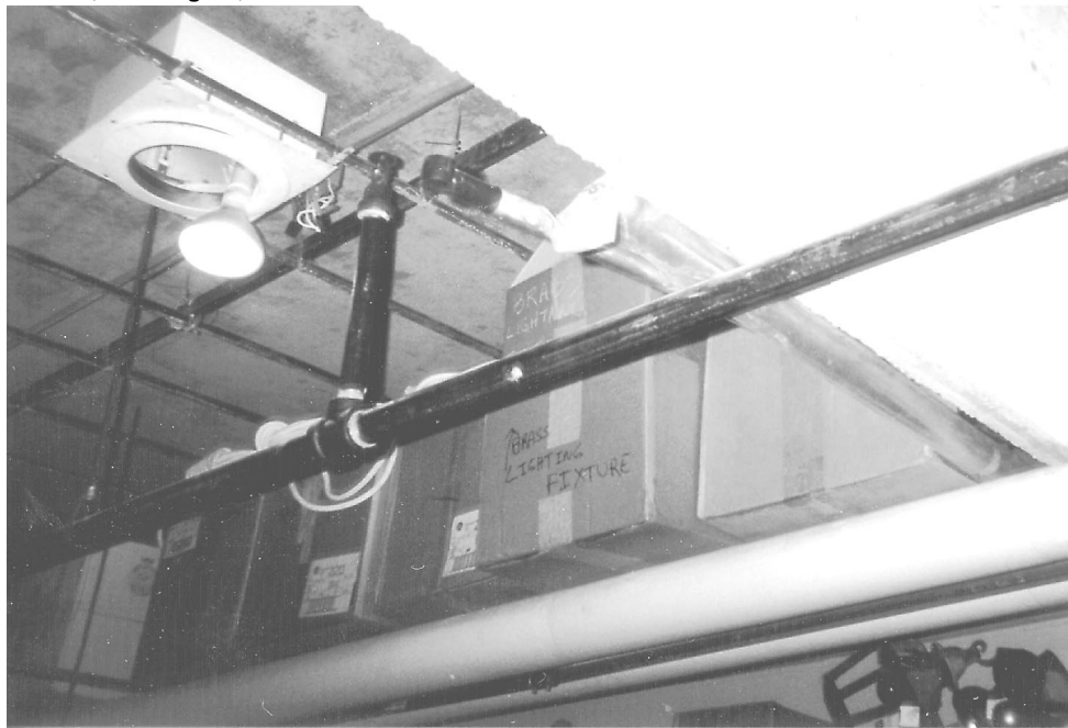
Figure 2: Boxes Impeding Effectiveness of Fire Sprinkler in Storage Area of the Ford National Theatre, Washington, D.C.
