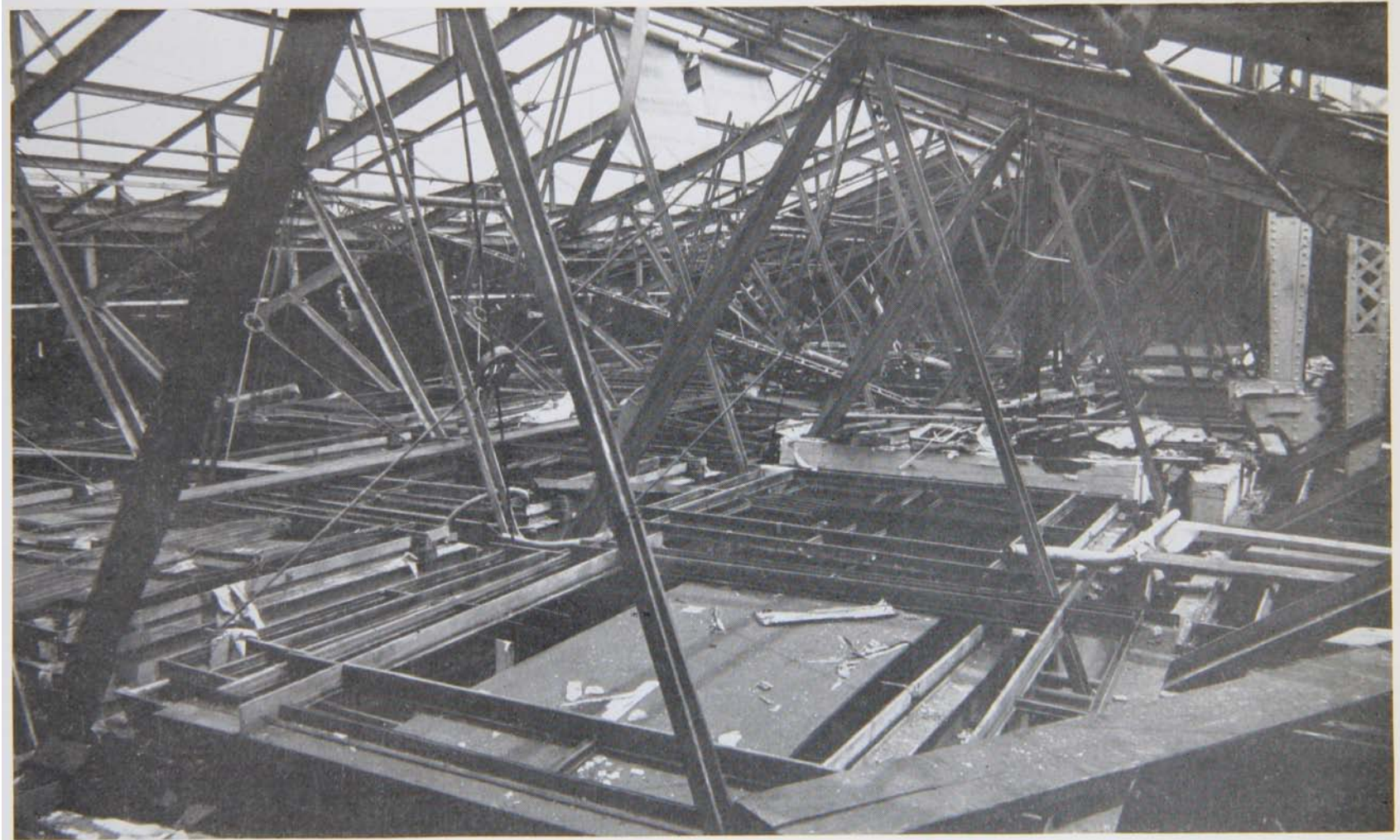
Old roof trusses and supporting steel for old skylights, from attic level, August 1, 1949.
