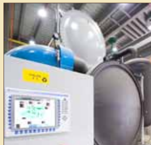
The U.S. Capitol Power Plant
