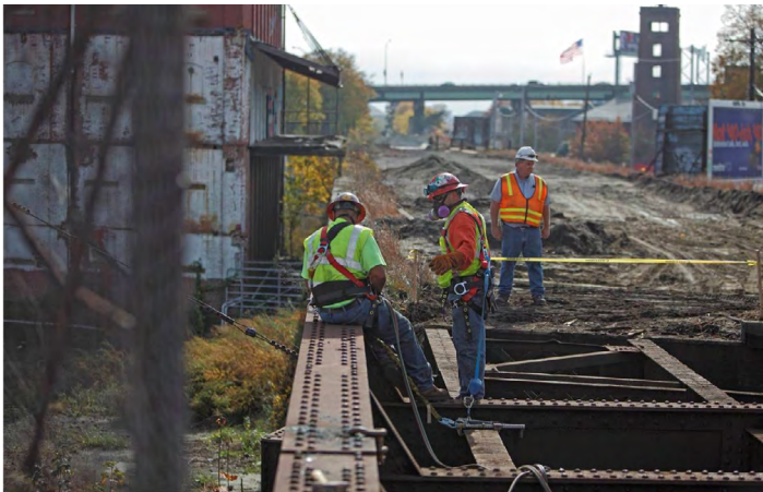
TIGER funds help reconstruct three freight rail bridges in New Bedford, MA
